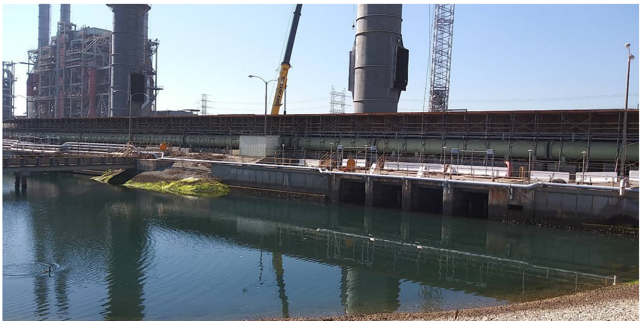
Photo 2. Southeast-facing view of proposed location for the new cooling tower on other side of wall. Haynes Intake Channel in foreground with demolished Unit 4 and Unit 5 stacks in background.
