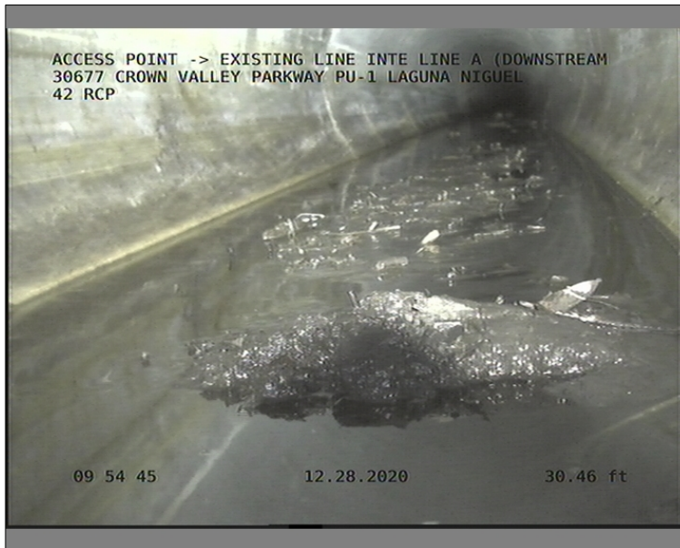
Photo: ACCESS POINT-EXISTING LINE INTERSECT-D-095336.JPG 30.46FT, Deposits Settled Other, 15 %of cross sectional area, from 05 to 07 o'clock, , within 8 inches of joint: YES
