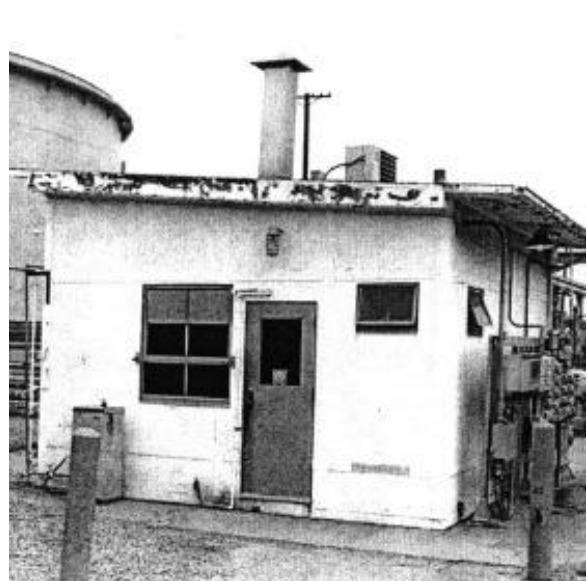
Figure 11: Substation, as it appeared in 2000. Jones & Stokes.
