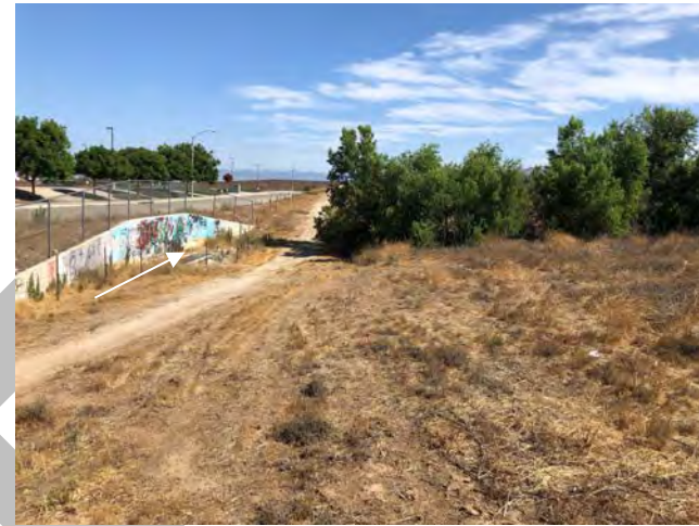
Photo 26. Overview of downstream extent of NWW-6, facing north, where NWW-6 drained into a storm drain inlet (white arrow) (33.900242, -117.313681). July 28, 2021.
