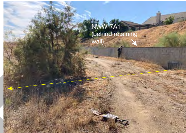
Photo 30. View of the upstream extent of NWW-7A (yellow dashed line), facing east, where flows from NWW-7A1 and NWW-7A2 travel through the culvert (33.898454, -117.313740). July 28, 2021.
