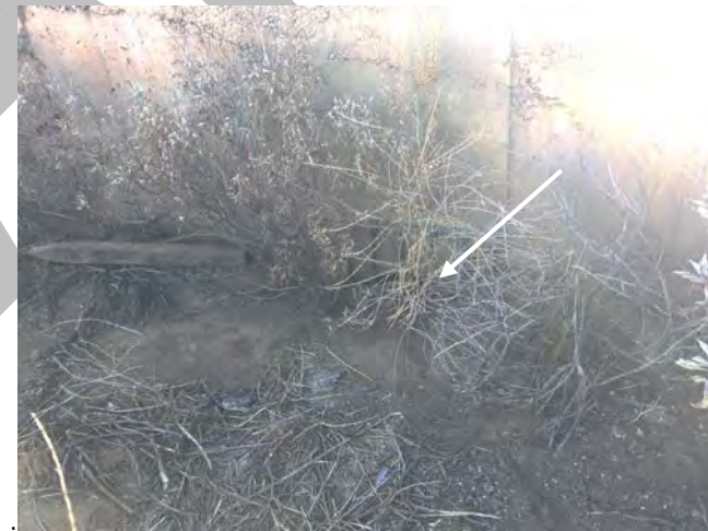
Photo 16. View of culvert (white arrow) blocked with sediment that historically received flows from AD-1, facing northeast (33.905876, -117.312380). August 6, 2021.
