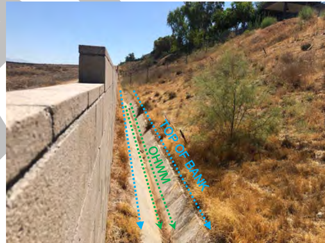
Photo 28. Upstream view of ODP 5 and view of WDP 2, facing east, within NWW-7A1. The OHWM was primarily defined by water staining. WDP 2 met the hydrology parameter; however, WDP 2 did not meet the hydrophytic vegetation or hydric soil parameters (33.898441, -117.313517). August 6, 2021.
