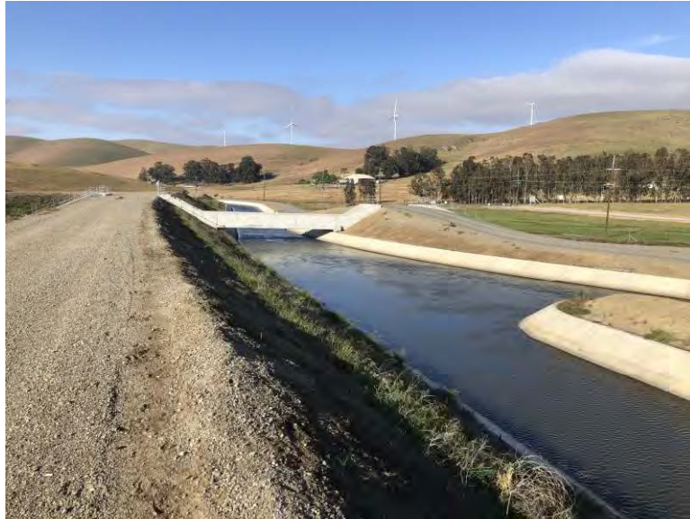
Figure 8. South Bay Aqueduct: Dyer segment, view looking south to confluence of Dyer Reservoir outlet canal and South Bay Aqueduct and overchute structure (IMG_5038)
