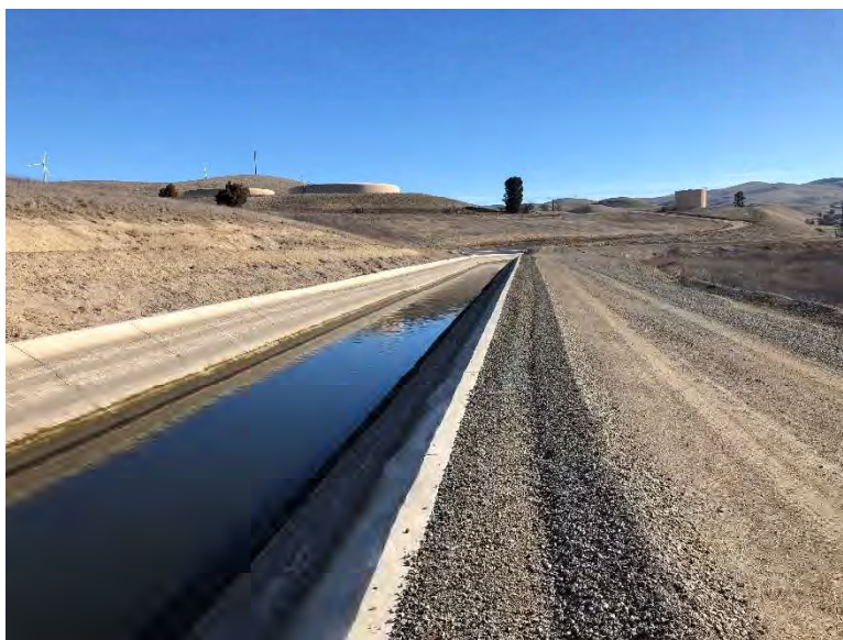
Figure 15. Patterson segment of South Bay Aqueduct, north of reservoir, view looking southeast (IMG_4179)
