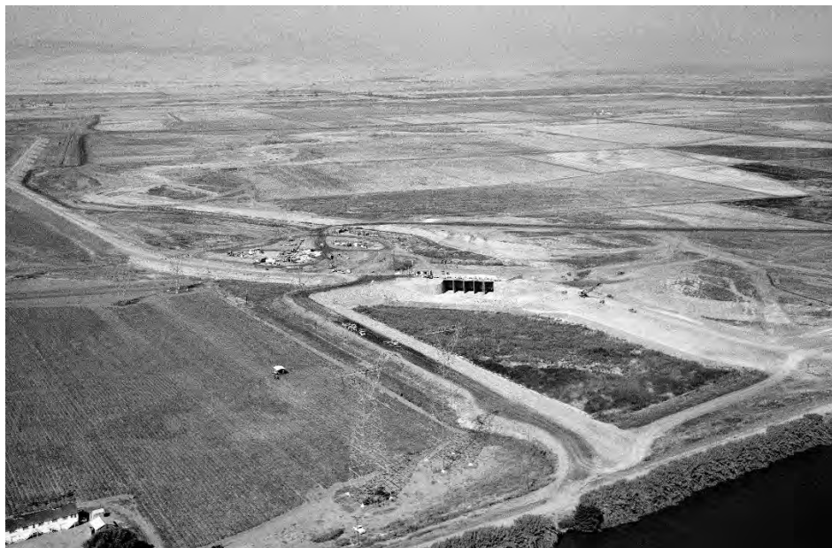
Exhibit D. 1969 aerial view looking northwest over the Clifton Court Forebay construction site showing the inlet structure and its five control gates in the foreground (DWR 1969).
