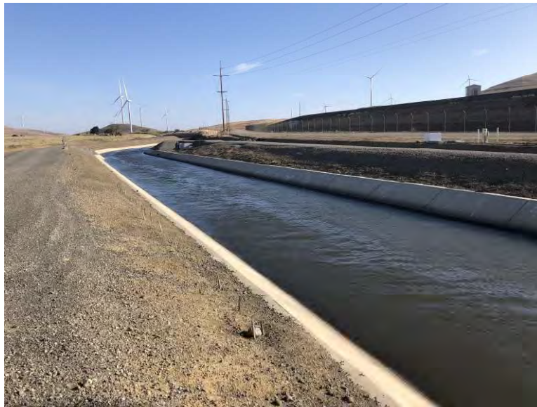
Figure 5. South Bay Aqueduct: Dyer segment, Dyer Reservoir in background, view looking northeast (IMG_4990)
