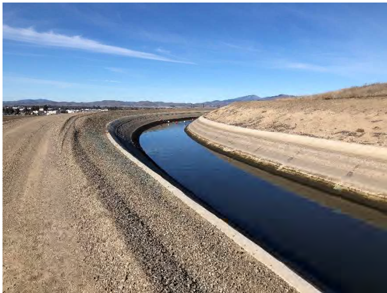
Figure 14. Patterson segment of South Bay Aqueduct, north of reservoir, view looking northwest (IMG_4178)
