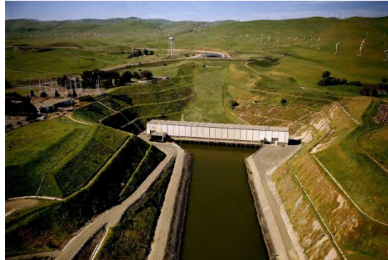
Photograph 17. Banks Pumping Plant. View to southwest. Source: Aquaforia, 2008.
