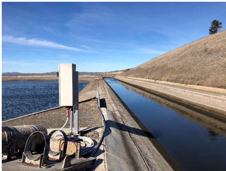
Figure 9. South Bay Aqueduct: Patterson segment, adjacent to Patterson Reservoir, view looking north (IMG_4128)
