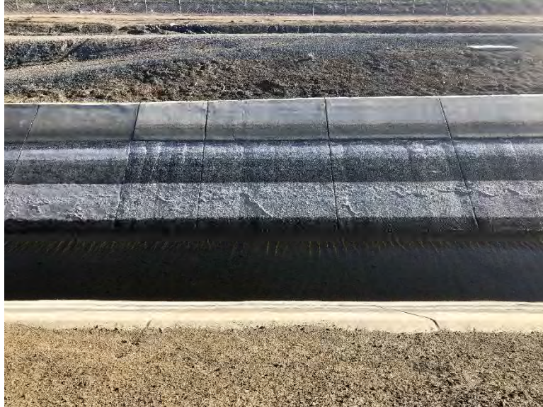
Figure 6. South Bay Aqueduct: Dyer segment near Dyer reservoir, view looking east (IMG_4066)
