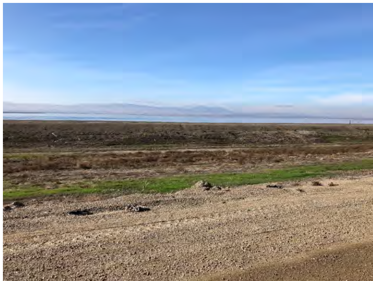
Figure 8. Clifton Court forebay, showing levee structure from access road, looking west (IMG_3949)
