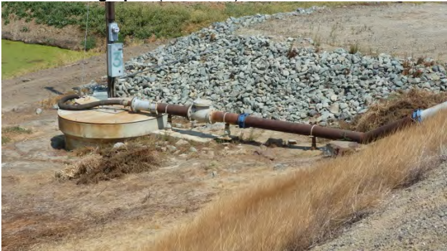
Photograph 2. Representative mechanical pump at Clifton Court Forebay. View to northwest.
