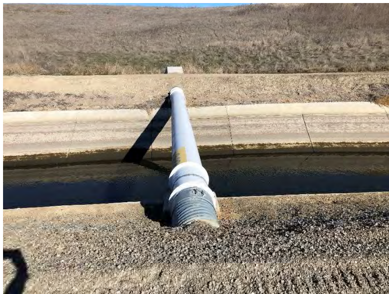
Figure 13. Patterson segment of South Bay Aqueduct, at modern pipe crossing, view looking northeast (IMG_4172)
