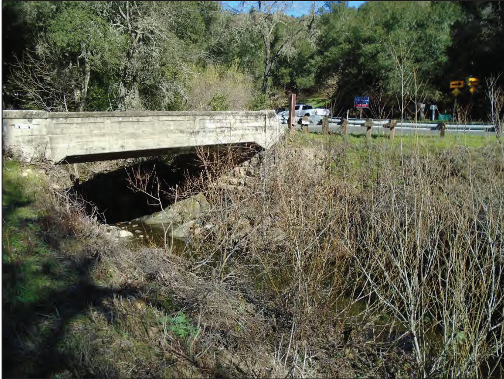
Figure 1. Dry Creek Bridge taken from the southwest bank of Dry Creek facing northeast; February 2018
