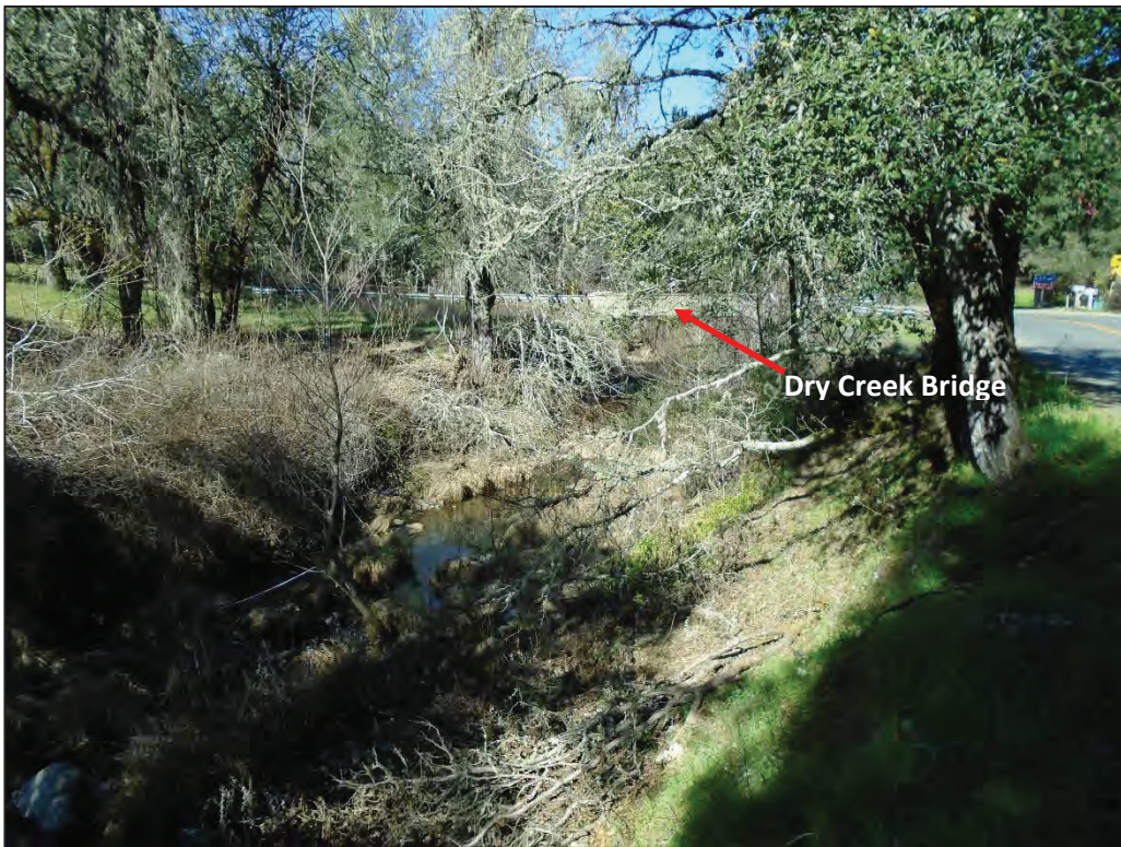
Figure 10. Dry Creek Bridge taken from the southeast bank of Dry Creek facing north; February 2018
