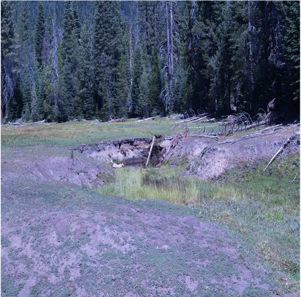
Photo 4: Overview of the 1.5-Meter-Deep Head Cut and Surrounding Impacted Area Note the significant amount of scour along both banks of the channel and the surface above.
