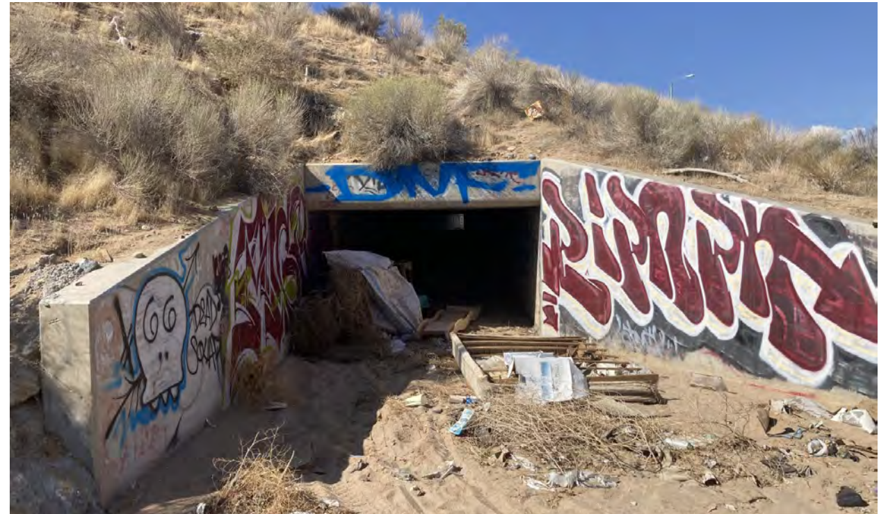
Photograph 4: Photo looking southwest within Drainage B near southern perimeter of the Project site. Photo depicts box culvert that conveys Drainage B beneath Ottawa Street.
