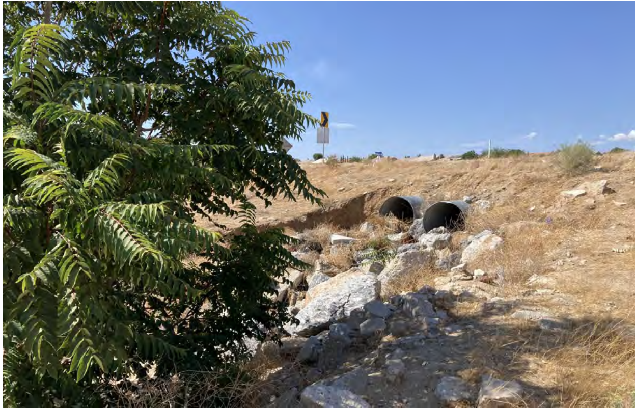
Photograph 1: Photo looking southwest (offsite) from western boundary of the Project site. Photo depicts piped culvert that conveys Drainage A beneath Hesperia Road.
