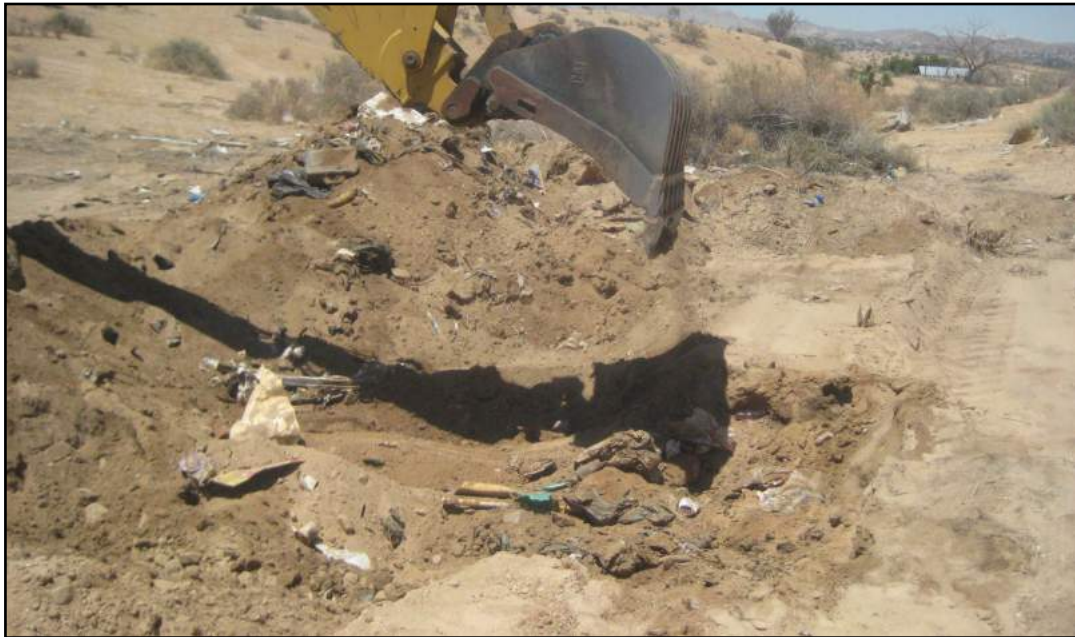
Photo 8—Removal and stockpiling of impacted soil and trash near northern end of flow path on parcel 551-07.
