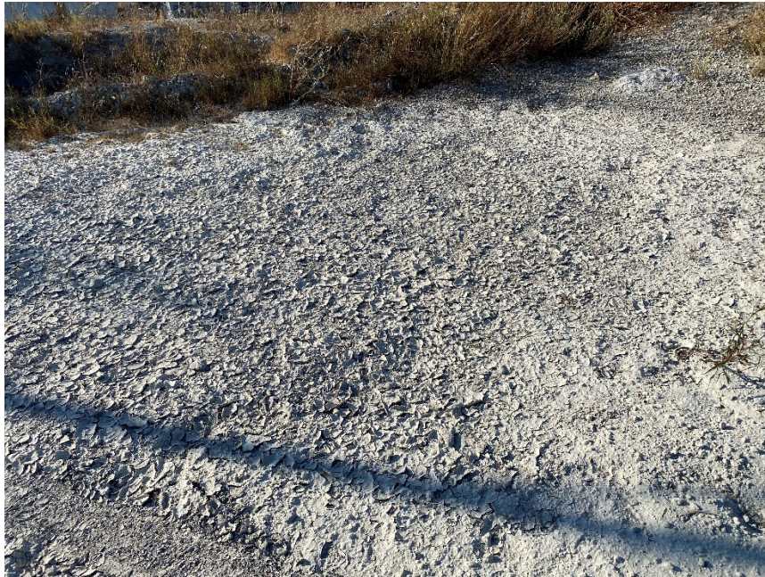
10. Photograph shows slight depression area along railroad spur terminus where water appears to pond during the rainy season; despite soil “flaking,” note absence of hydrophytic vegetation.
