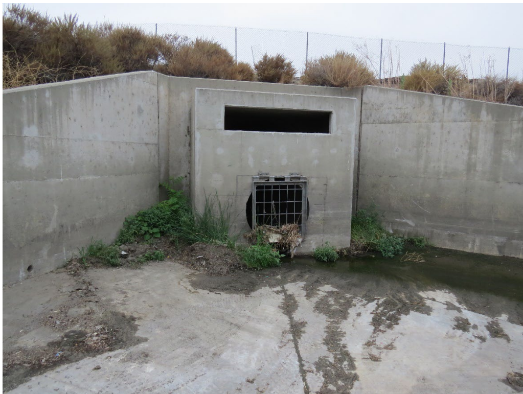
Photograph 12: A culvert in the water detention basin in the southwest corner of the project site that conveys flows off-site to San Sevaine Channel.
