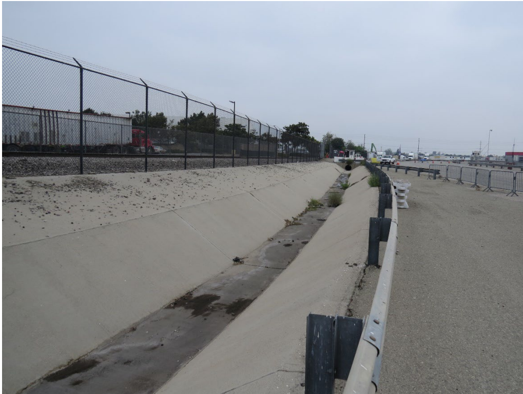
Photograph 13: A concrete v-ditch that flows along the southwestern portion of the project site.
