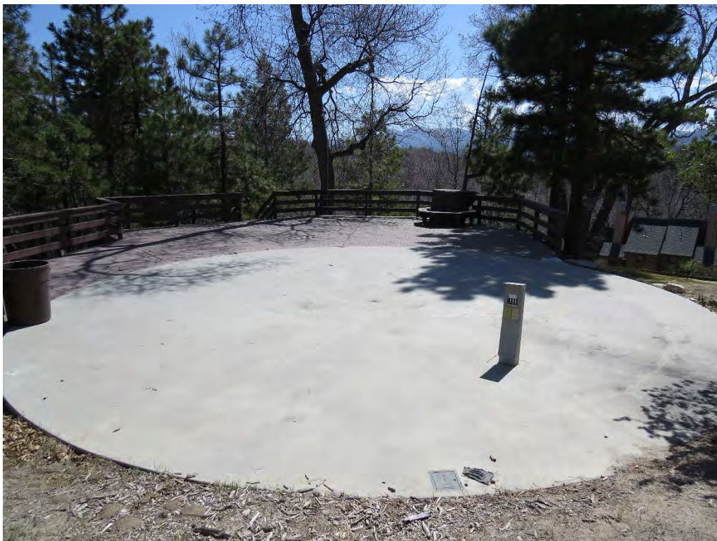
Photograph 12: Existing platform and concrete area where a gazebo was located on the middle of the eastern portion of the survey area.
