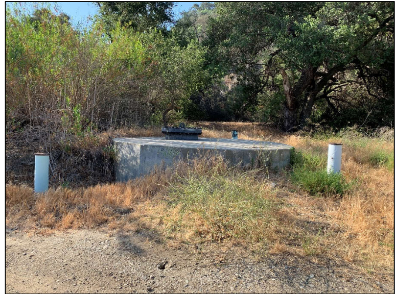
b. Structure W-A, valves buried under exposed vertical pipes
