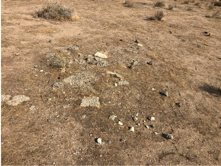
Concrete debris in north end of site. View to northwest.
