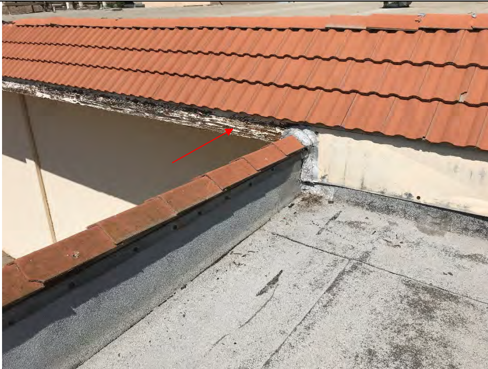
Photo #9 View of roofing (HA #07) at 325 Hampshire Road, Unit B-F. This material is an ACM. Beige paint at wood trim is lead-based paint (LBP; see red arrow).
