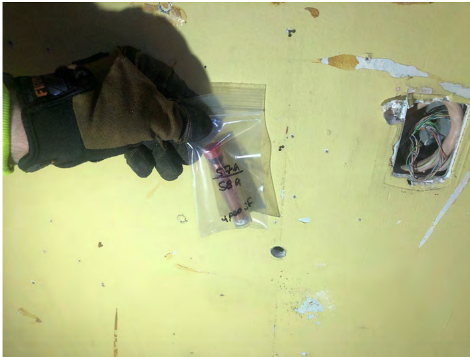
Photo #17 View of wall system within 325 Hampshire Road, Unit D. The joint compound (HA #58) is an ACM.
