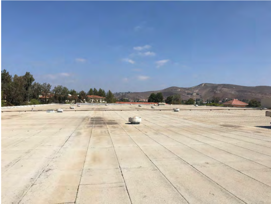
Photo #5 View of across the roof of 325 Hampshire Road, Unit A, looking north.
