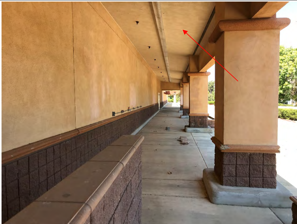
Photo #10 View of stucco (HA #21) at slanted overhang at 325 Hampshire Road, Unit A. This material is an asbestos-containing construction material (ACCM; see red arrow).
