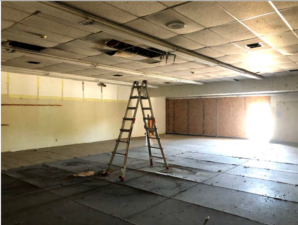
Photo #11 View of wall system within 325 Hampshire Road, Unit F. The joint compound (HA #40) is an ACM.
