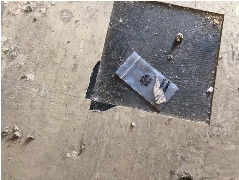
Photo #15 View of pale gray/green 12" x 12" VFT (HA #53) and associated mastic (HA # 54) within 325 Hampshire Road, Unit E. The VFT and mastic are ACMs.
