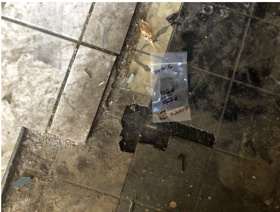
Photo #22 View of cream/yellow adhesive (HA #77) associated with gray/white faux marble pattern VFT within 325 Hampshire Road, Unit C. This material is an ACM.
