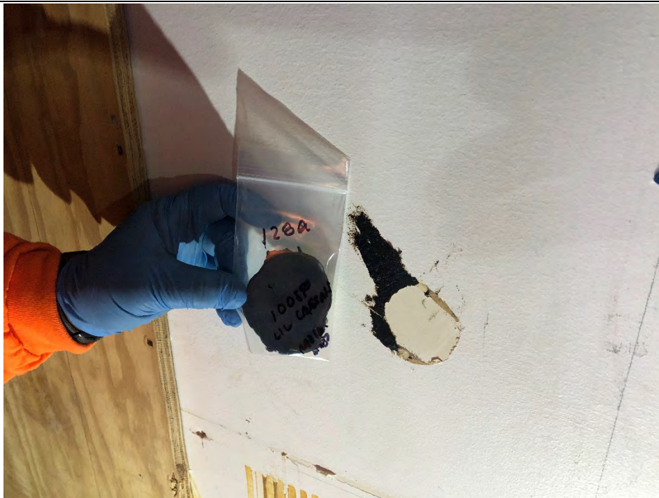
Photo #33 View of black residual mirror adhesive (HA #128) on walls within the former dining area of 325 Hampshire Road, Unit A. This material is an ACM.
