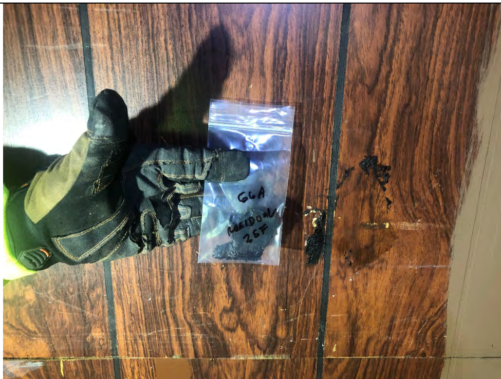
Photo #18 View of black residual mirror adhesive (HA #66) within 325 Hampshire Road, Unit D. This material is an ACM.
