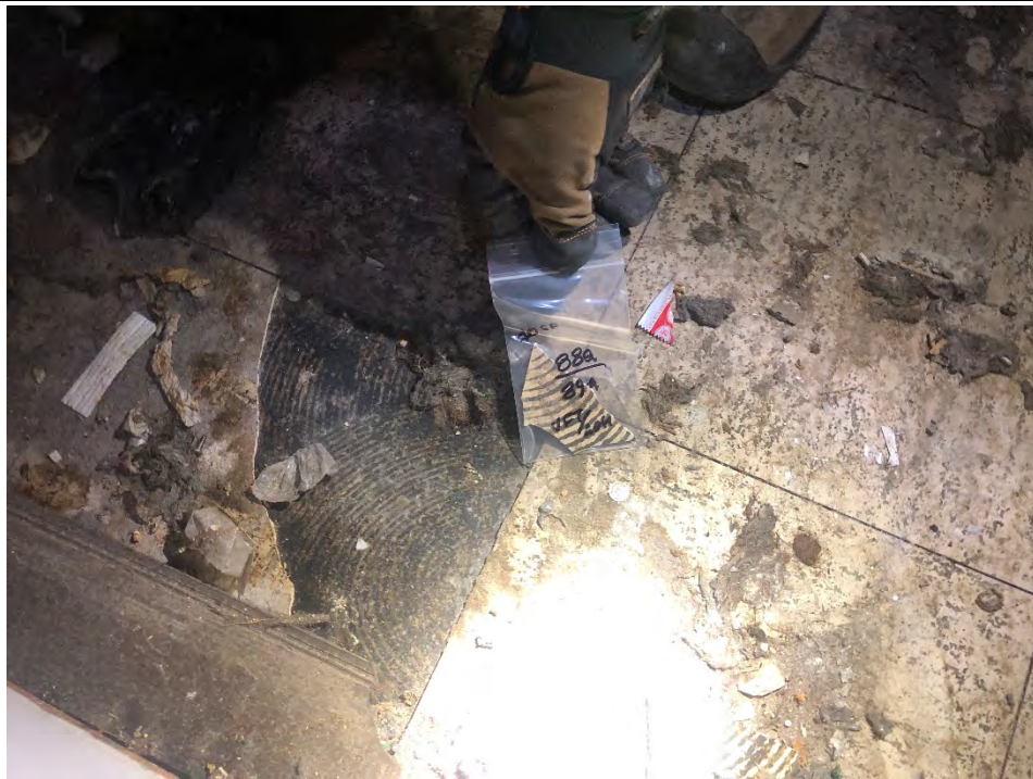
Photo #25 View of gray/brown 12" x 12" VFT (HA #88) and associated adhesive (HA #89) concealed beneath ceramic tile within 325 Hampshire Road, Unit C. The VFT and adhesive are ACMs.
