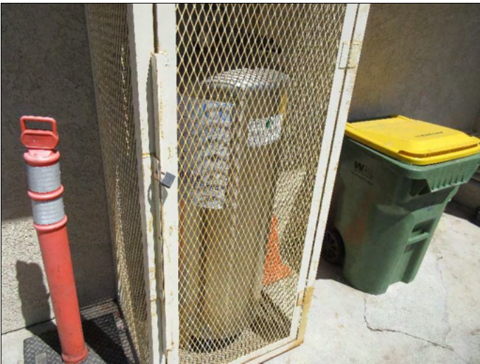
15. View of CO2 tank
