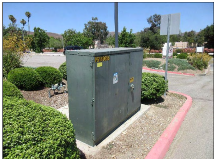
18. View of onsite transformer
