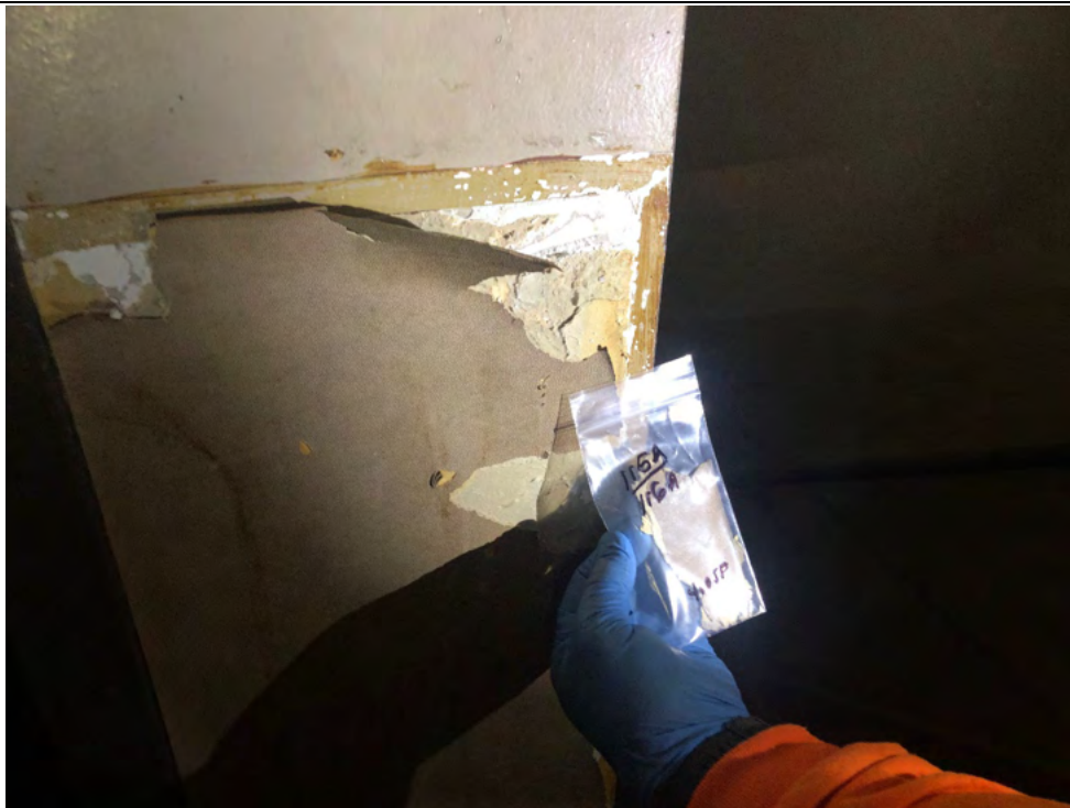
Photo #32 View of wallpaper (HA #115) in hallway outside Room #106 within 325 Hampshire Road, Unit A. The wallpaper is concealing a layer of joint compound (HA #116 – joint compound layer). The joint compound is and ACCM.
