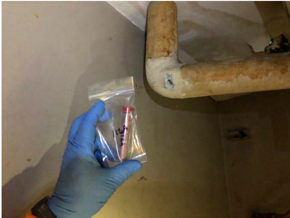
Photo #31 View of thermal system insulation (TSI) pipe elbow (HA #112) within 325 Hampshire Road, Unit A. This material is an ACM.
