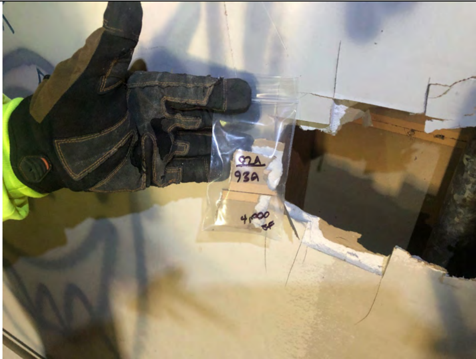
Photo #27 View of wall system within 325 Hampshire Road, Unit B. The joint compound (HA #93) is an ACM.
