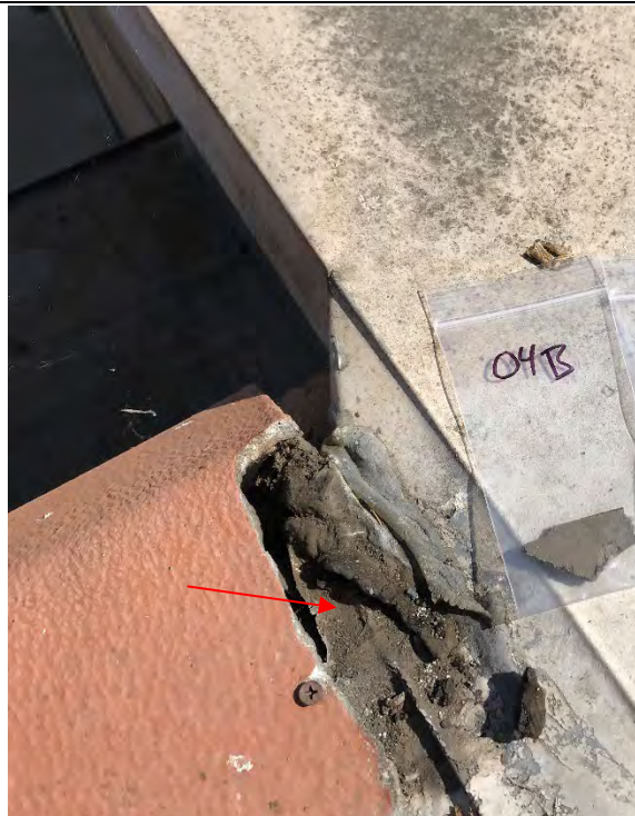
Photo #8 View of black paper (HA #04) beneath terra cotta tile at the roof of 325 Hampshire Road. This material is an ACM (see red arrow).
