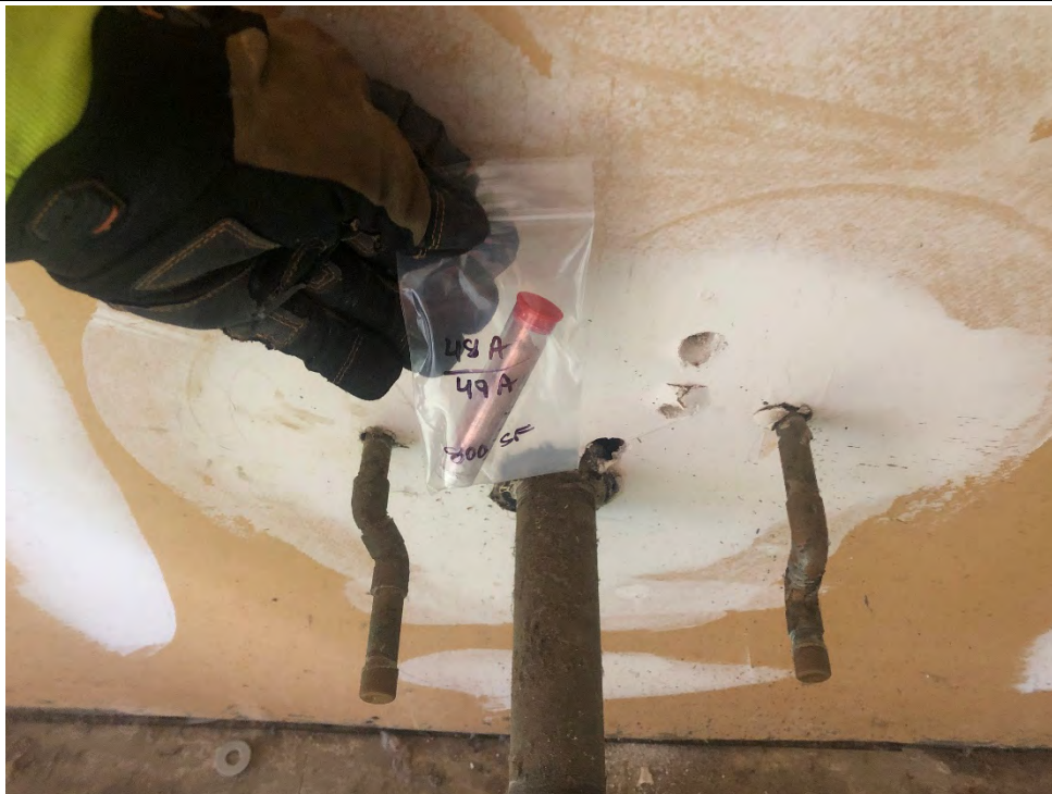
Photo #14 View of wall system within 325 Hampshire Road, Unit E. The joint compound (HA #49) is an ACM.
