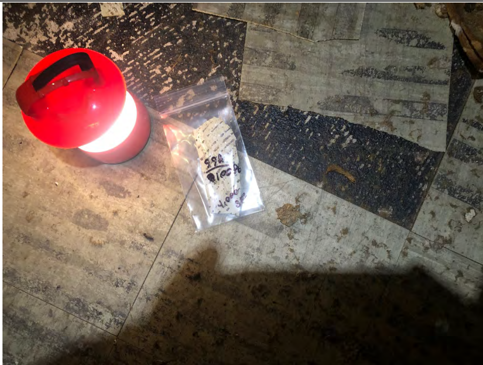
Photo #28 View of gray-green 9" x 9" VFT (HA #99) and associated mastic (HA #100) within 325 Hampshire Road, Unit B. The VFT and mastic are ACMs.
