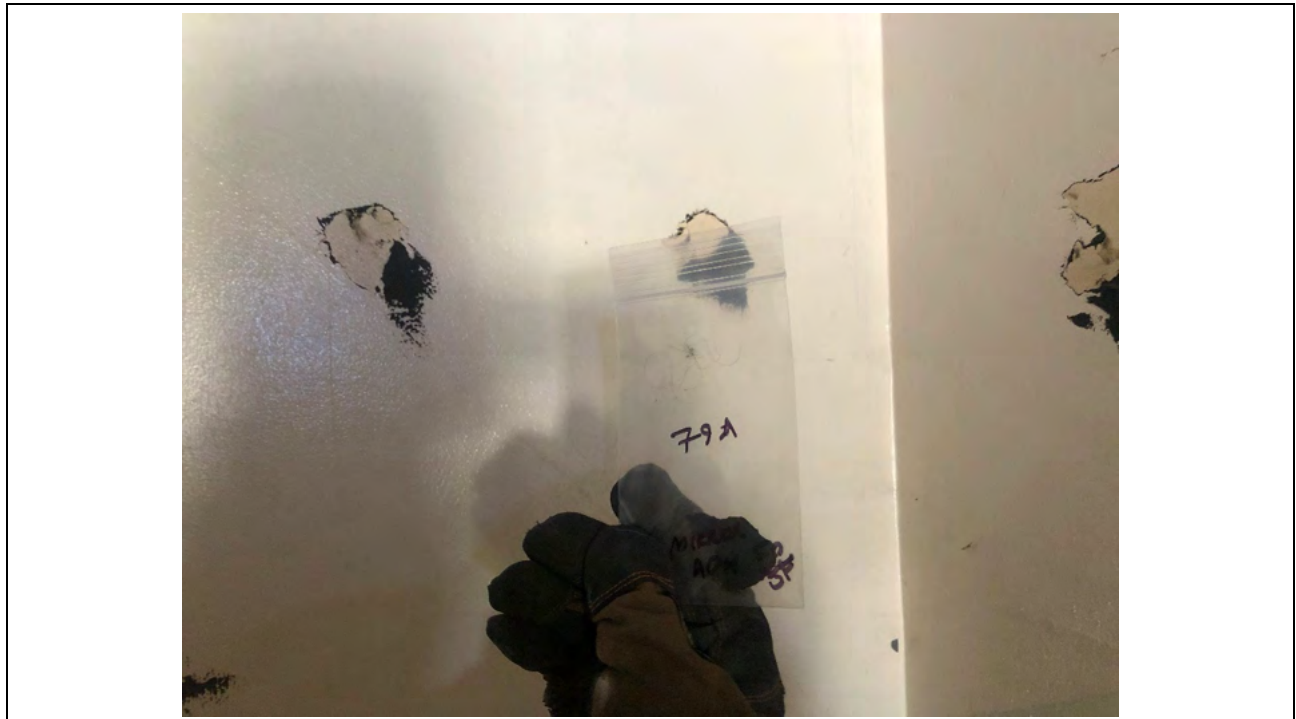
Photo #23 View of black residual mirror adhesive (HA #79) within 325 Hampshire Road, Unit C. This material is an ACM.
