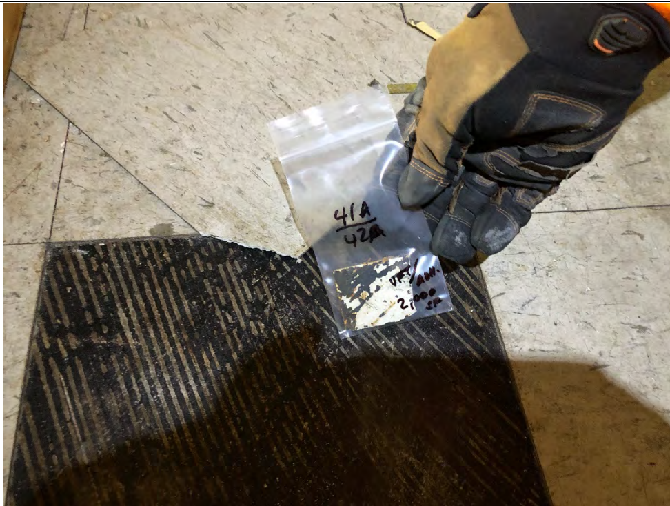
Photo #12 View of cream 12" x 12" vinyl floor tile (VFT; HA #41) and associated mastic (HA # 42) within 325 Hampshire Road, Unit F. The VFT and mastic are ACMs.
