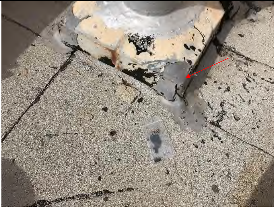
Photo #7 View of gray/black sealant (HA #03) at the roof of 325 Hampshire Road. This material is an asbestos-containing material (ACM; see red arrow).
