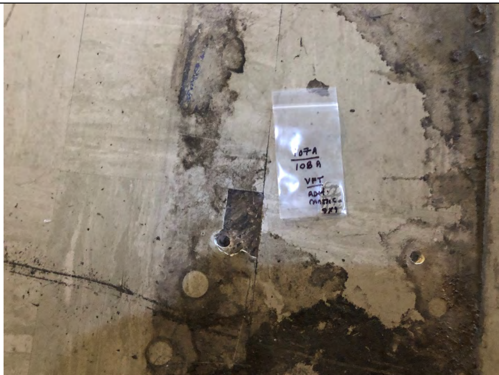
Photo #30 View of pale gray/green 9" x 9" VFT (HA #107) and associated mastic (HA #108) within 325 Hampshire Road, Unit A. The VFT and mastic are ACMs.
