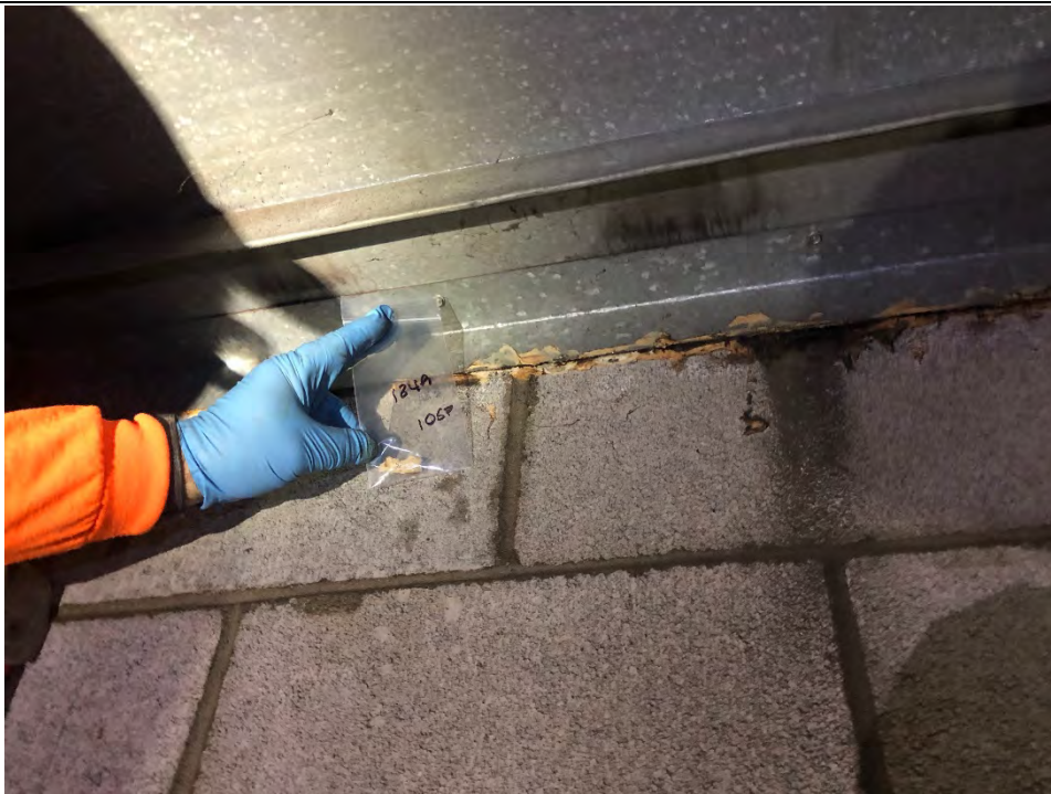
Photo #35 View of yellowish-white caulking (HA #134) at air handlers within the west central equipment room of 325 Hampshire Road, Unit A. This material is an ACM.
