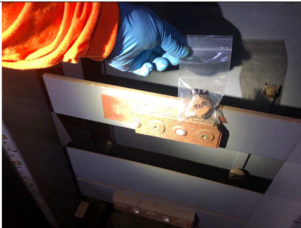
Photo #34 View of electrical insulation board (HA #132) at electrical panel within 325 Hampshire Road, Unit A. This material is an ACM.
