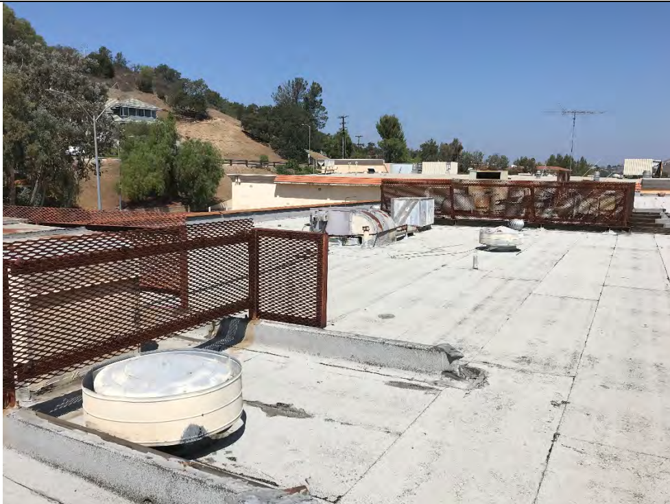
Photo #6 View of across the roof of 325 Hampshire Road, Unit A-F, looking northwest.
