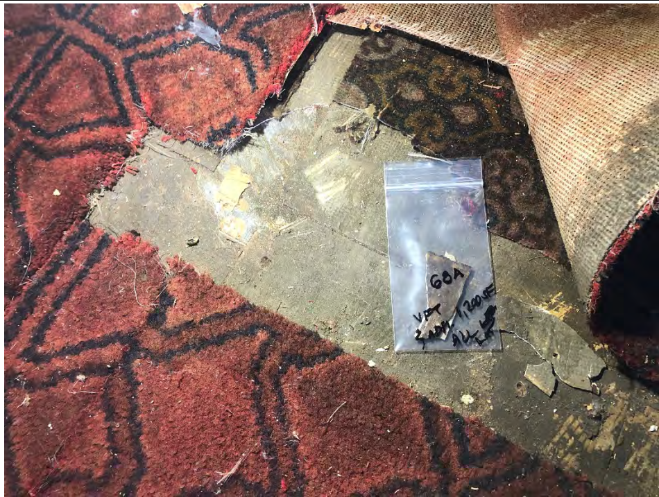
Photo #19 View of multi-layer white/brown VFT (HA #68) within 325 Hampshire Road, Unit D. This material is an ACM.
