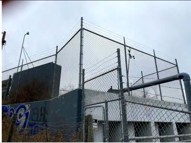
Storm lift station on northern side of property.
