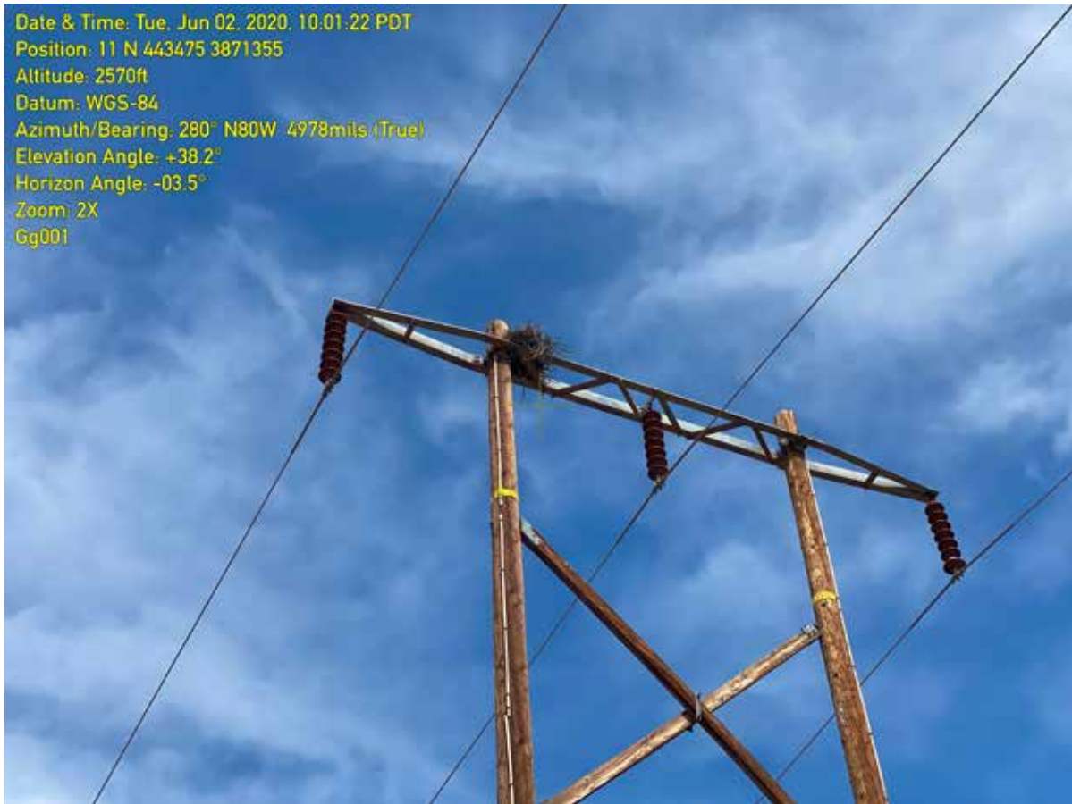
Photograph 4. Raven nest on cross member in existing structure near Aratina gen-tie
