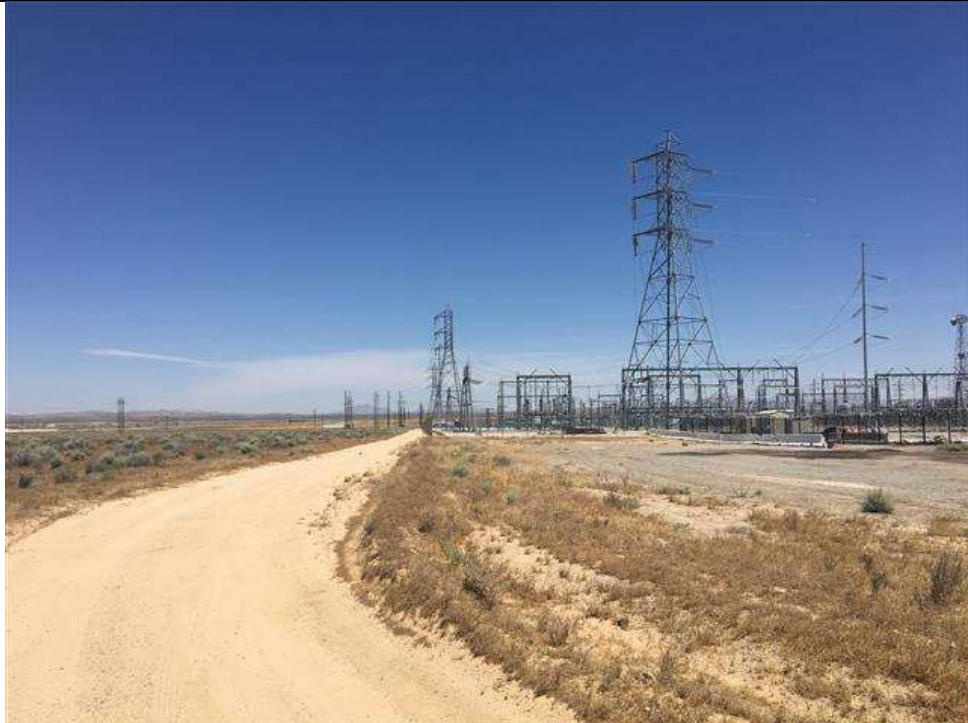
Photo #21 Facing north near the SCE Kramer substation (Figure 7).
