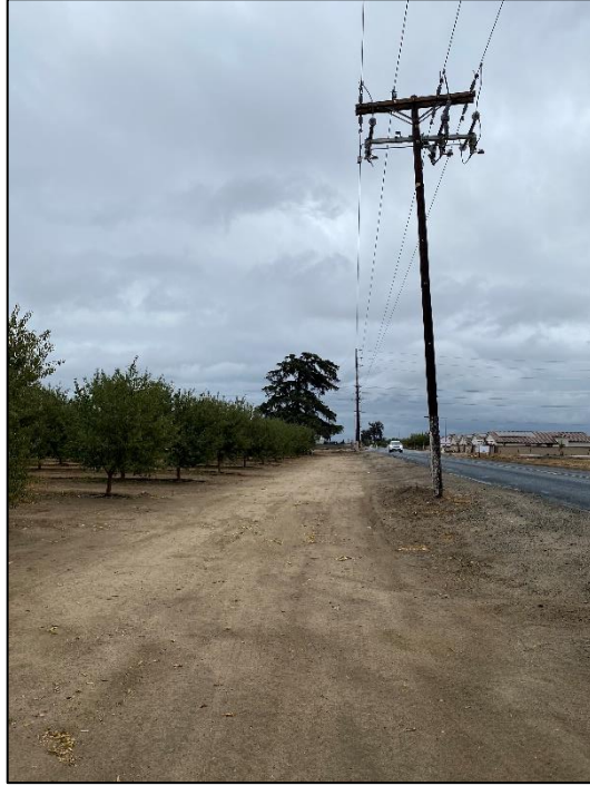
Figure 4-5 Wooden distribution line on north side of West Riggan Ave, facing east.
