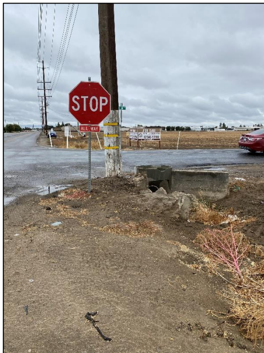
Figure 4-4 Dirt ditch and concrete culvert at northwest corner of West Riggin Ave and North Shirk Road, facing south.
