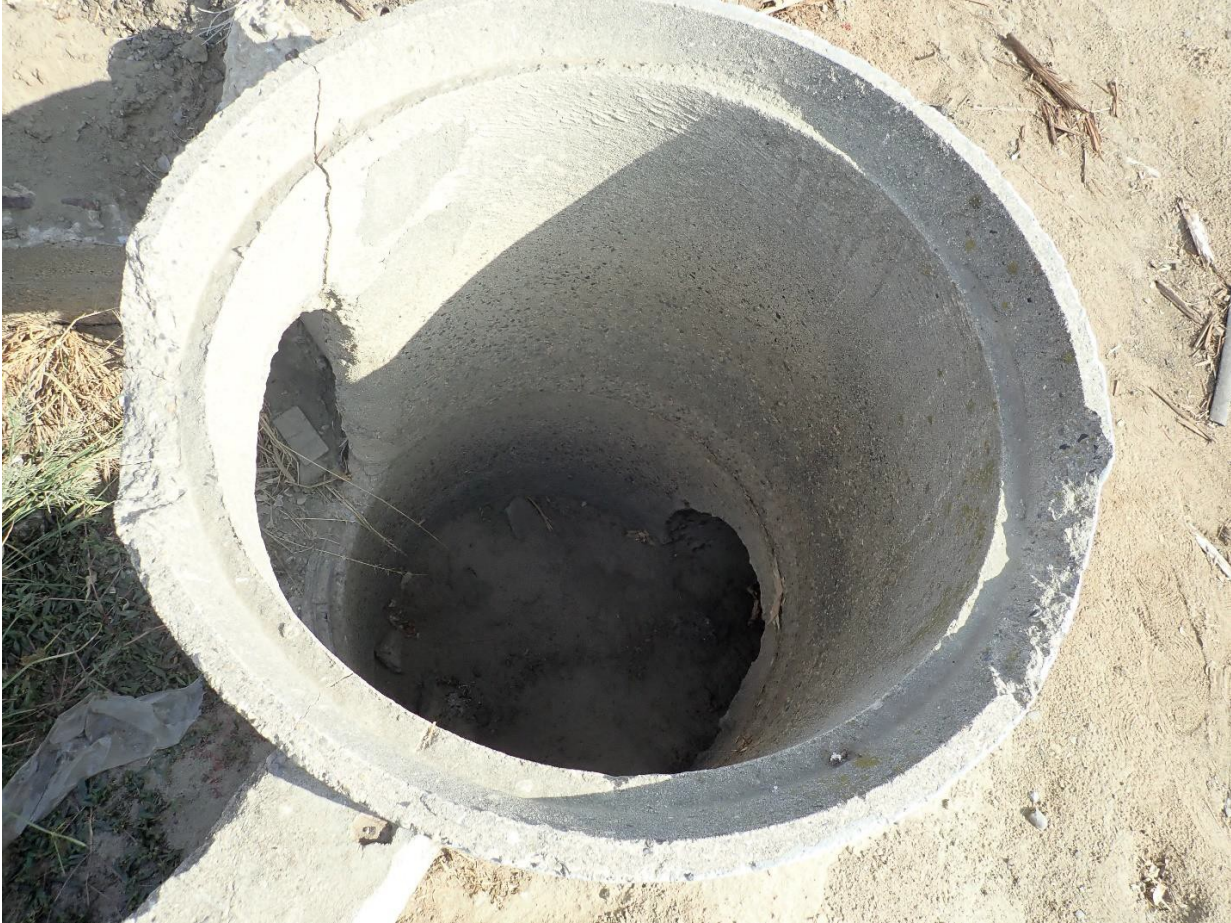
Figure 7 – Concrete irrigation culvert located on the northwestern corner of Shirk St at Riggin Ave, the culvert traverses north to south under Riggin Avenue at intersection with Shirk Street (Facing northeast)
