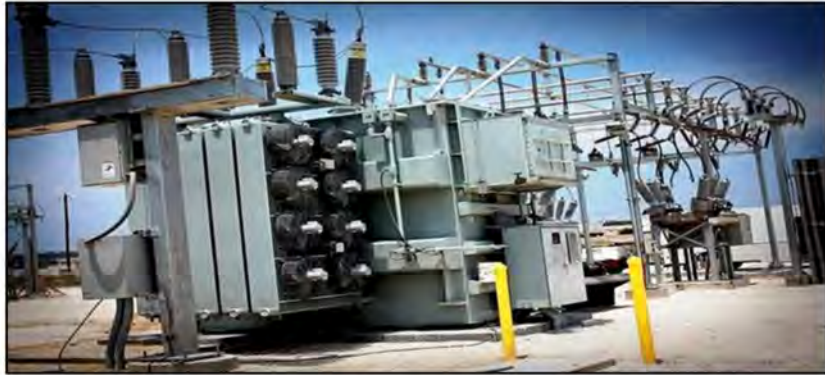
Example of Transformers (on left) and Circuit/Tie Breakers (on right) located on concrete pads. Transformers approximately 30 feet by 50 feet; circuit/tie breakers approximately 10 feet by 12 feet.
