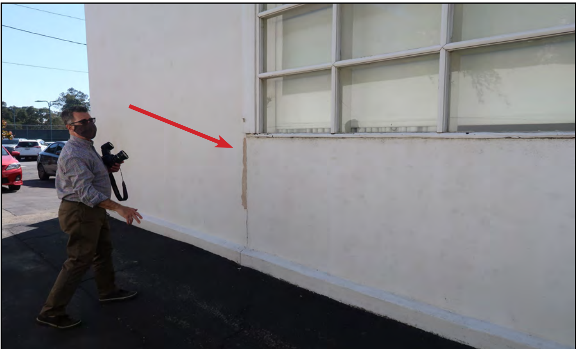
Image 11: Detail of steel sash window on east elevation, note the tear in stucco where window originally extended to ground level and infilled at a unknown date, view southwest (Chattel, 2021)
