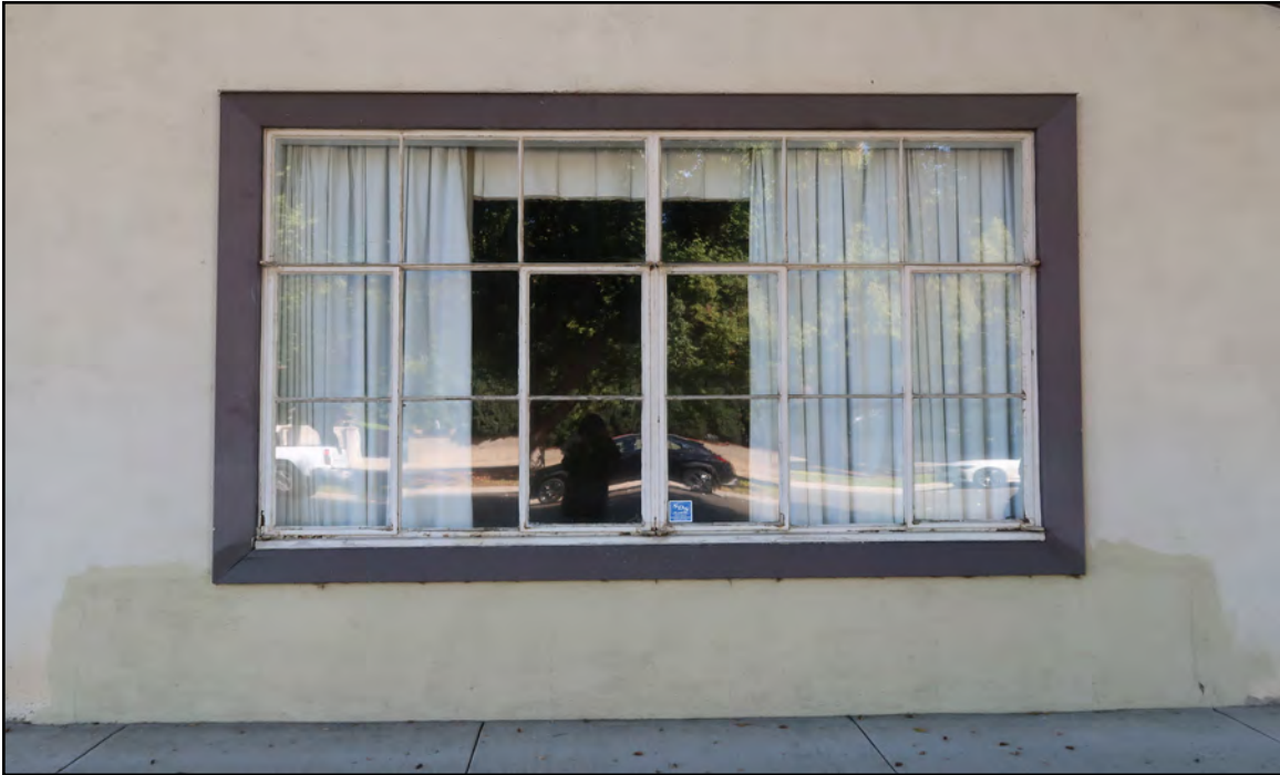
Image 5: San Marino Center, north elevation, note steel sash windows with wooden bevel frame, view south (Chattel, 2021)
