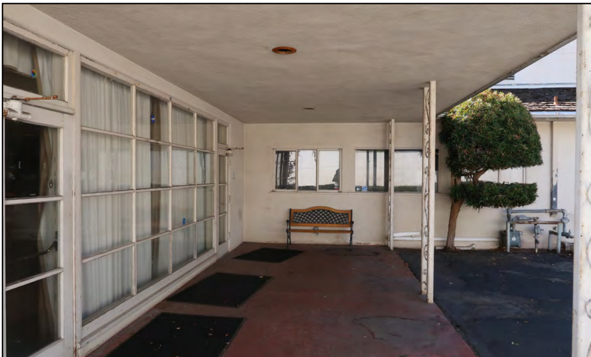
Image 9: Detail of recessed porch on east elevation, note steel sash windows and original wooden doors, view west (Chattel, 2021)
