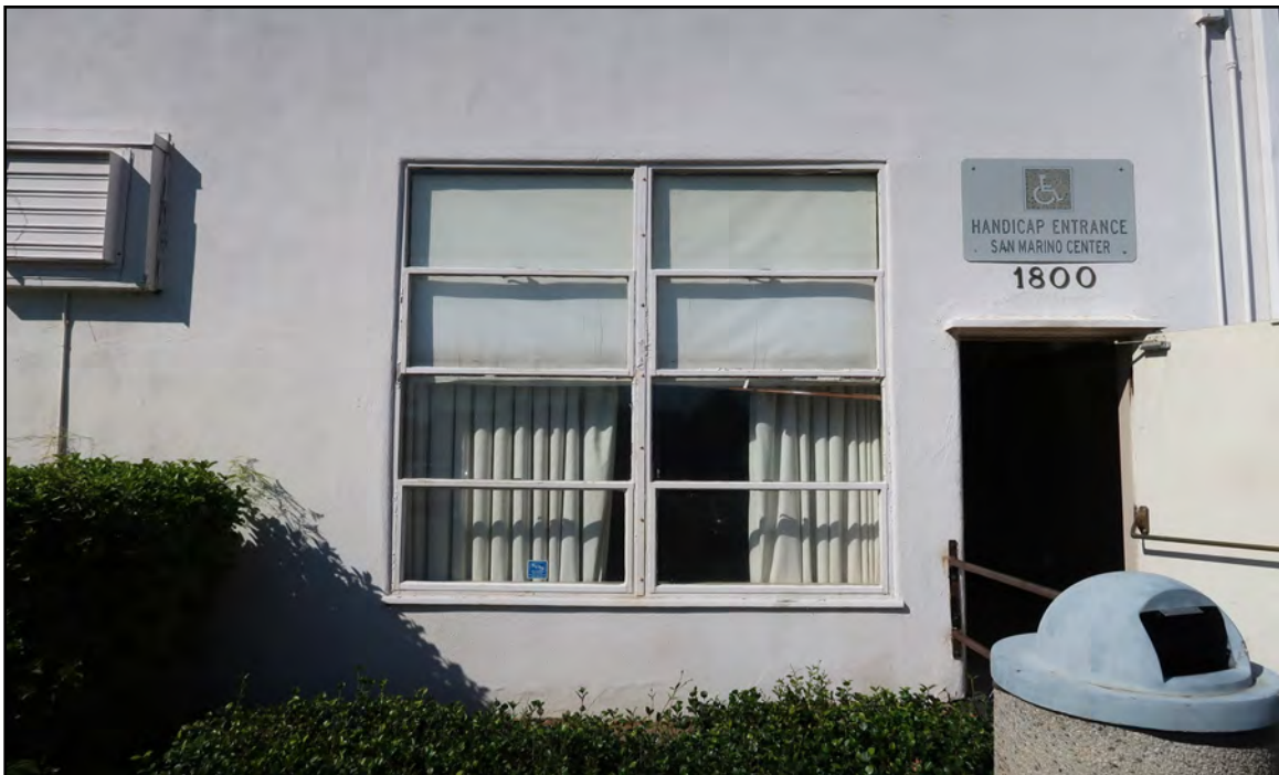
Image 13: Detail of steel sash window on the south elevation, view north (Chattel, 2021)
