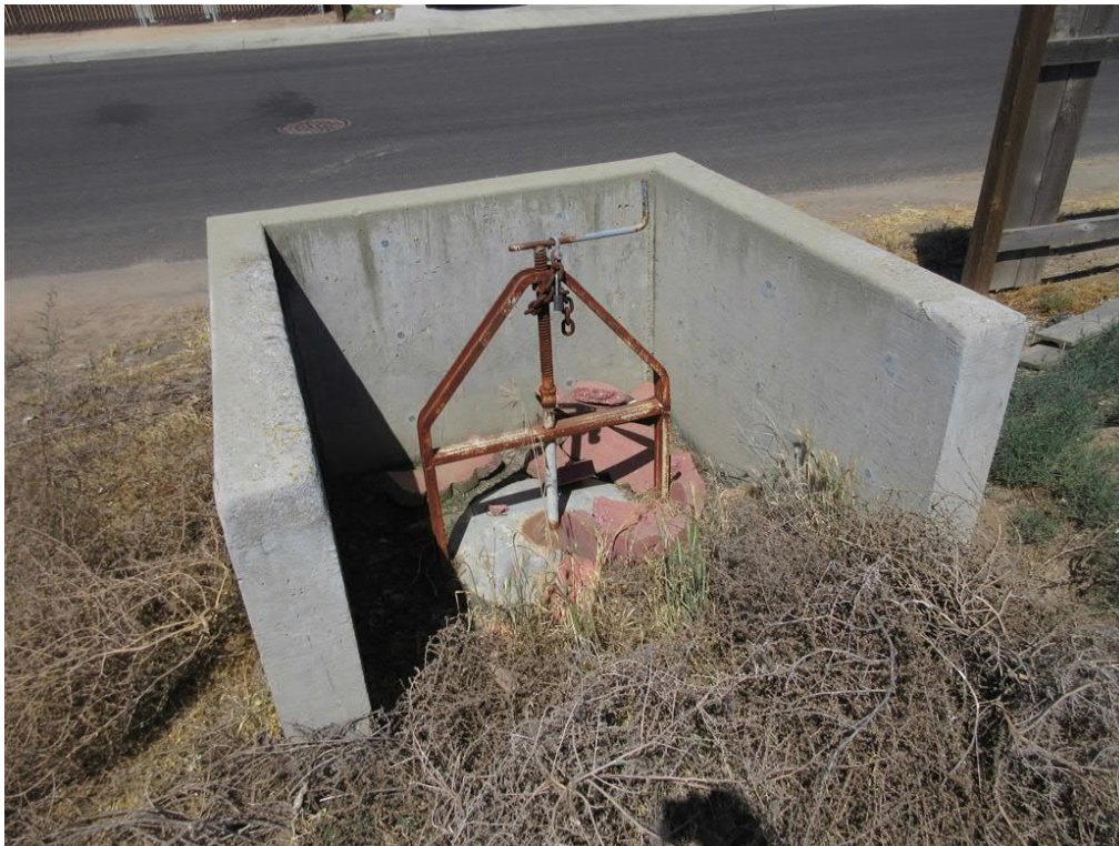
Photo 10: View of a representative irrigation system capture box located in the western portion of the subject site.
