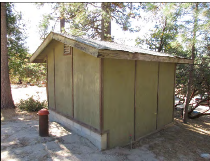
17. Existing inactive water pump house and active water well located at the eastern end of the subject property
