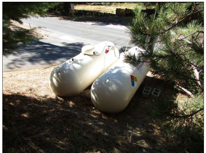
12. Two 500-gallon aboveground propane tanks located in the northwest corner of the subject property
