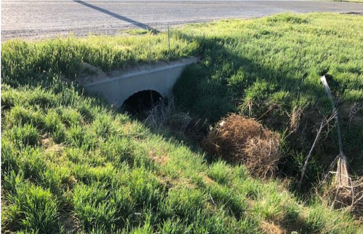
Photograph 7. Showing where the erosional drainage feature meets the culvert under Spruce Avenue.
