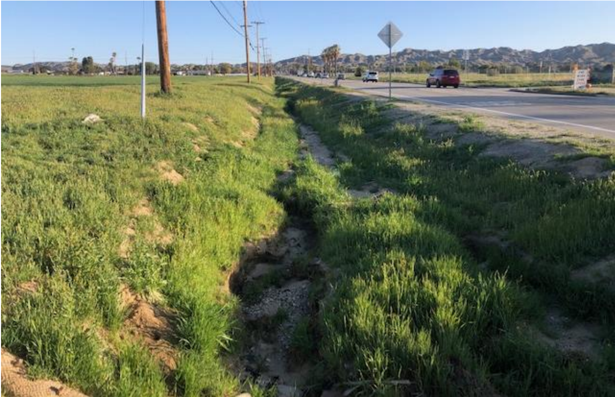
Photograph 1. Facing north west of Redlands Boulevard looking at the roadside drainage ditch.
