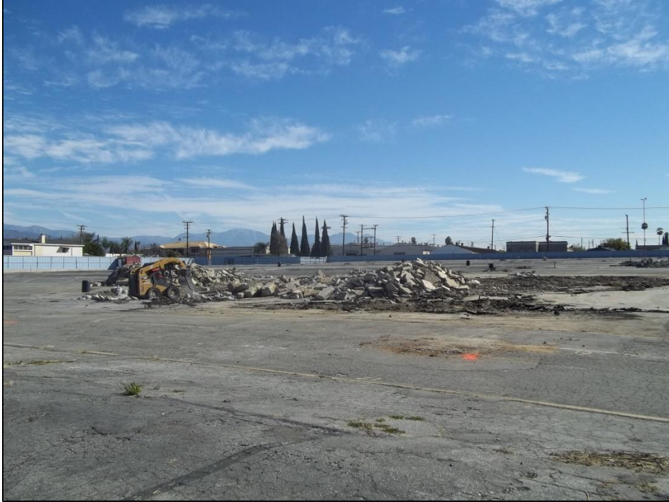
E-7. Location of Starlite Drive-In theater concessions stand and projection room (demolished), facing northeast
