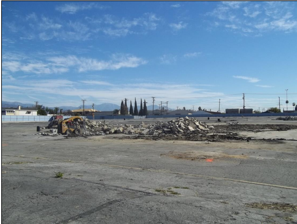
7. Location of Starlite Drive-In concessions stand and projection room (demolished), facing northeast
