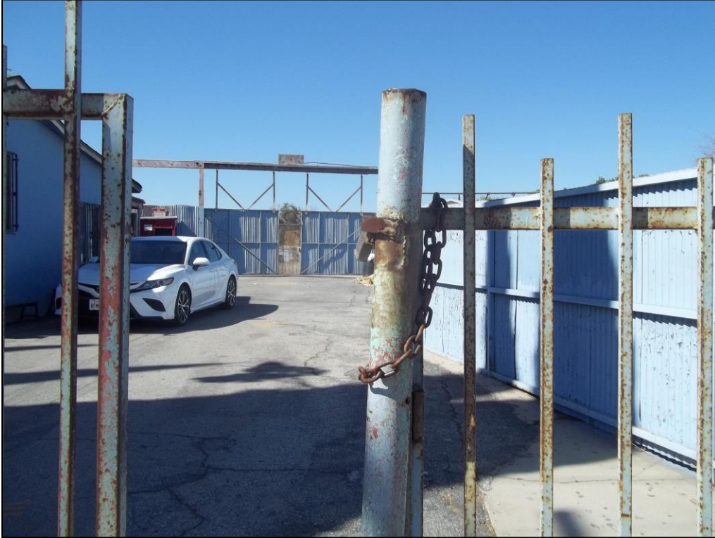
Starlite Drive-In theater access gate at the western boundary of the residential property, facing west
