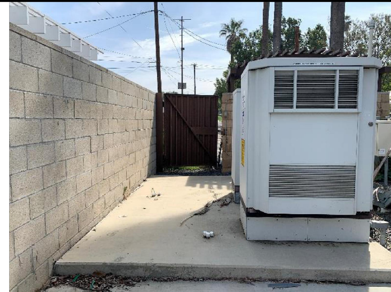
View of Inside Cell Site Panoramic #3
