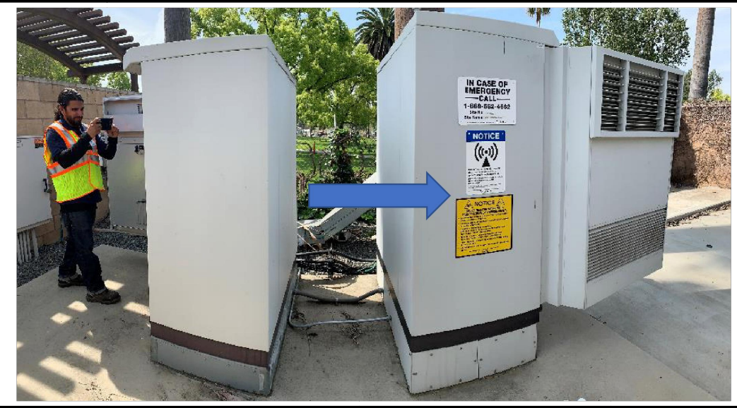
View of Power Source (BTS)
