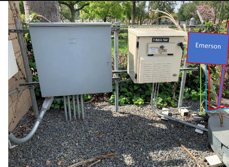
View of Fiber, Power and Ground Conduit Path
