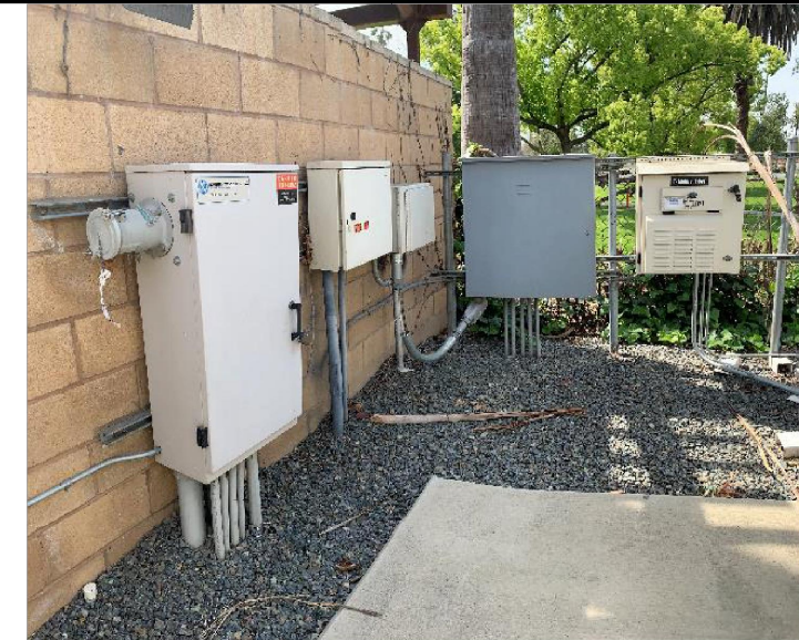
View of Inside Cell Site Panoramic #4
