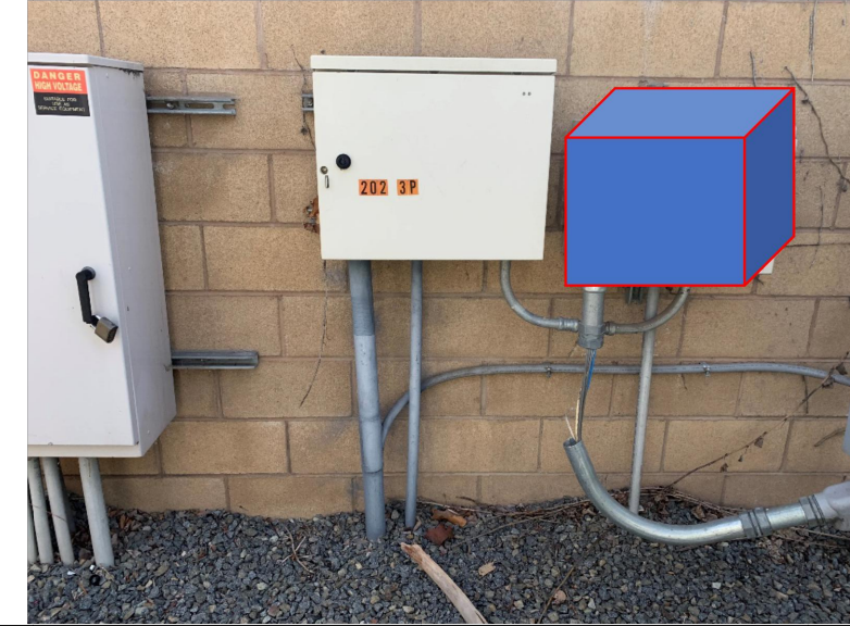
View of (N) 12x12x8 Telco Box
