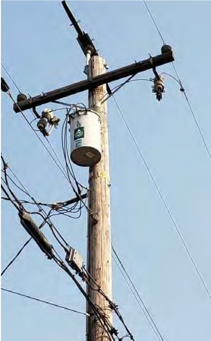
Photo 33: Pole-mounted transformer across Irwin Avenue from residence; note non-PCB sticker on transformer.
