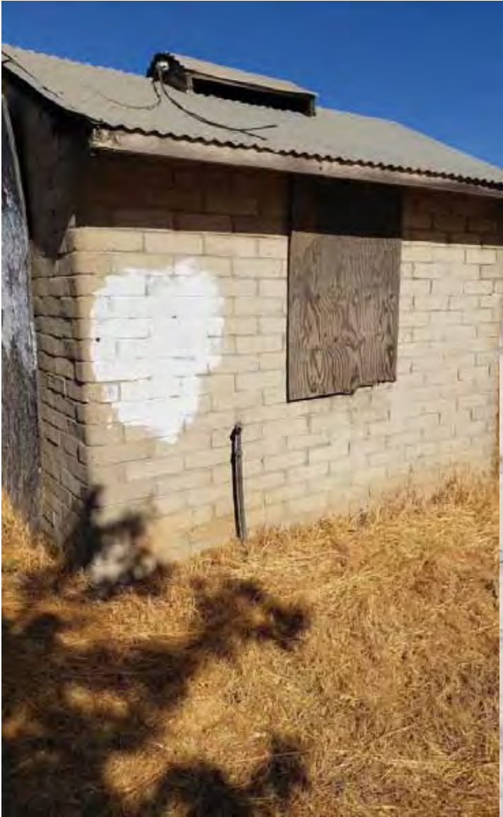
Photo 7: Boarded up pump house
