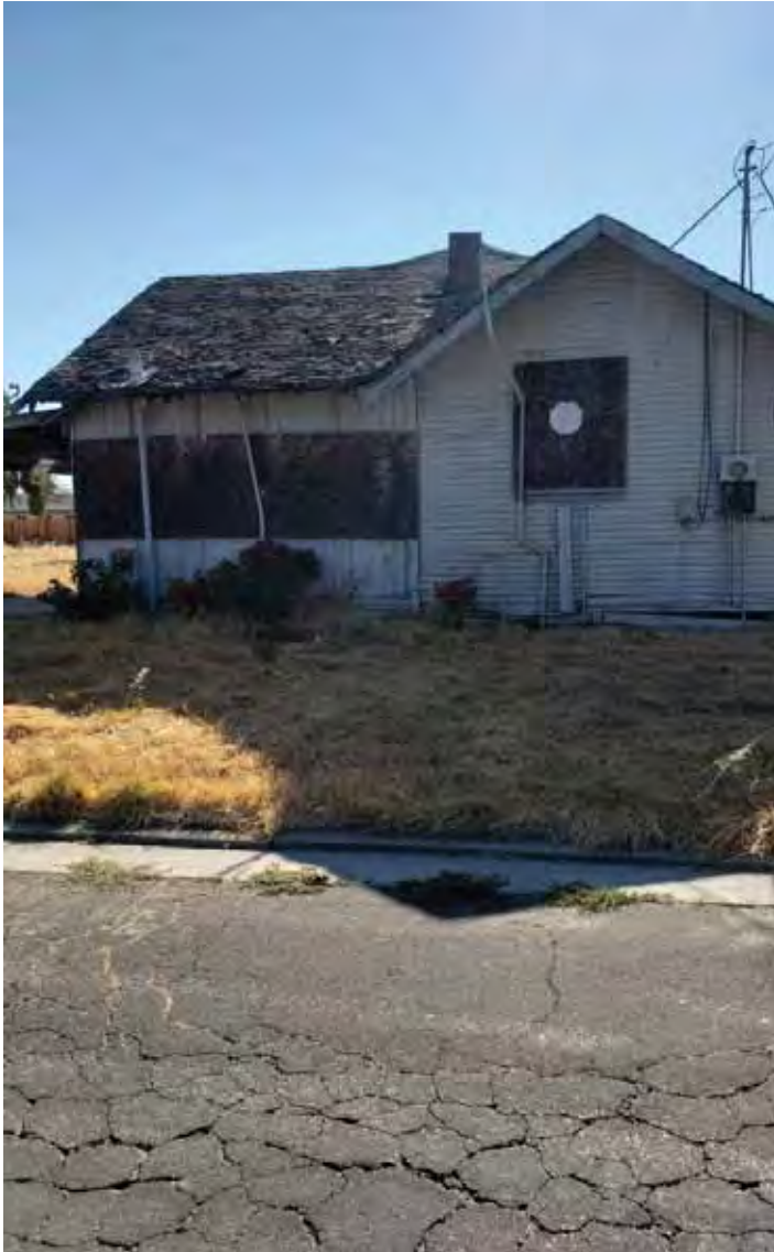
Photo 13: West side of boarded up residence.
