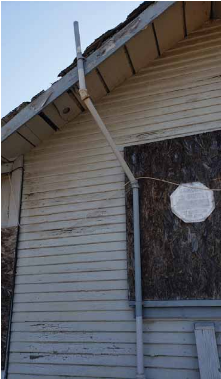
Photo 15: Apparent vent line on west side of residence.
