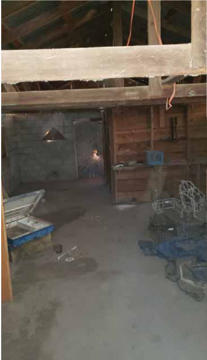
Photo 5: Photo taken through space above locked garage door.
