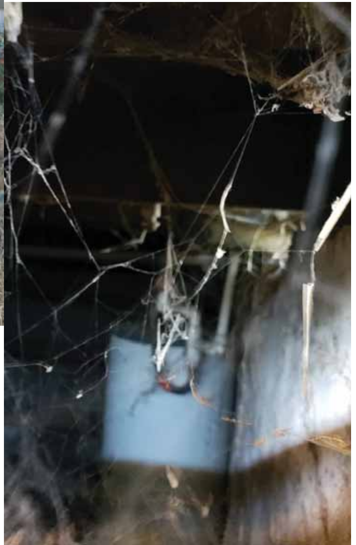
Photo 18: Photo inside cellar, taken from outside through space between floor of the building and the plywood barrier blocking the cellar entrance.
