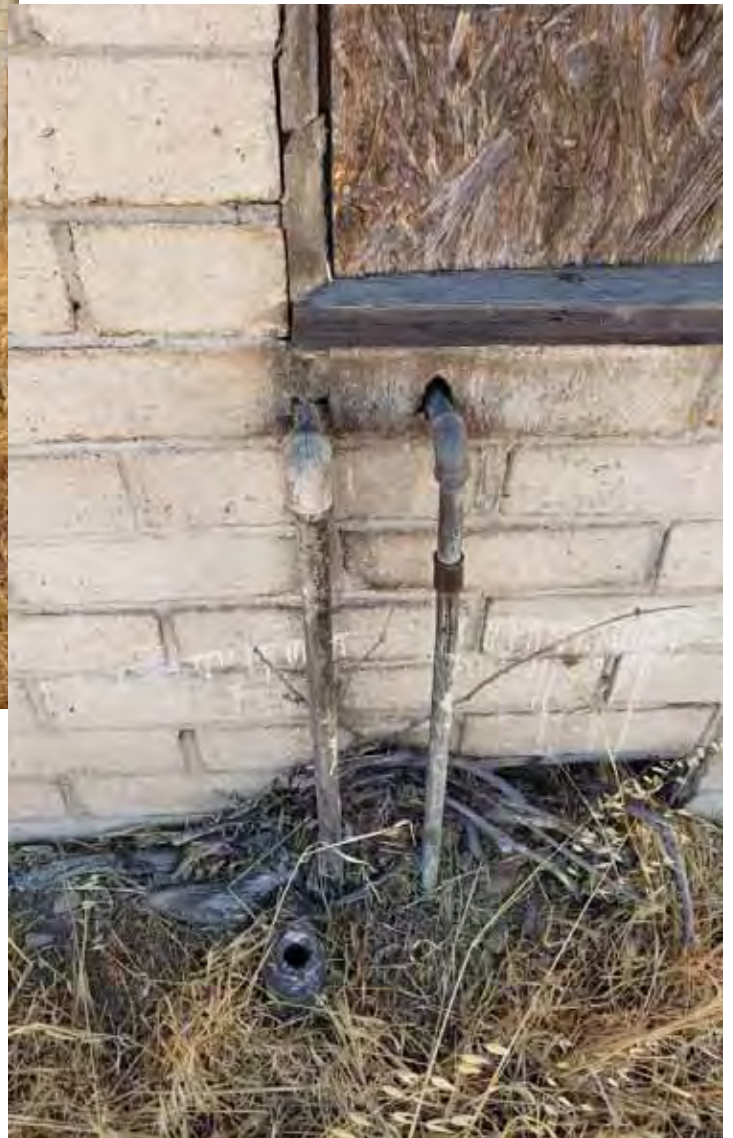
Photo 8: Piping on west side of pump house.
