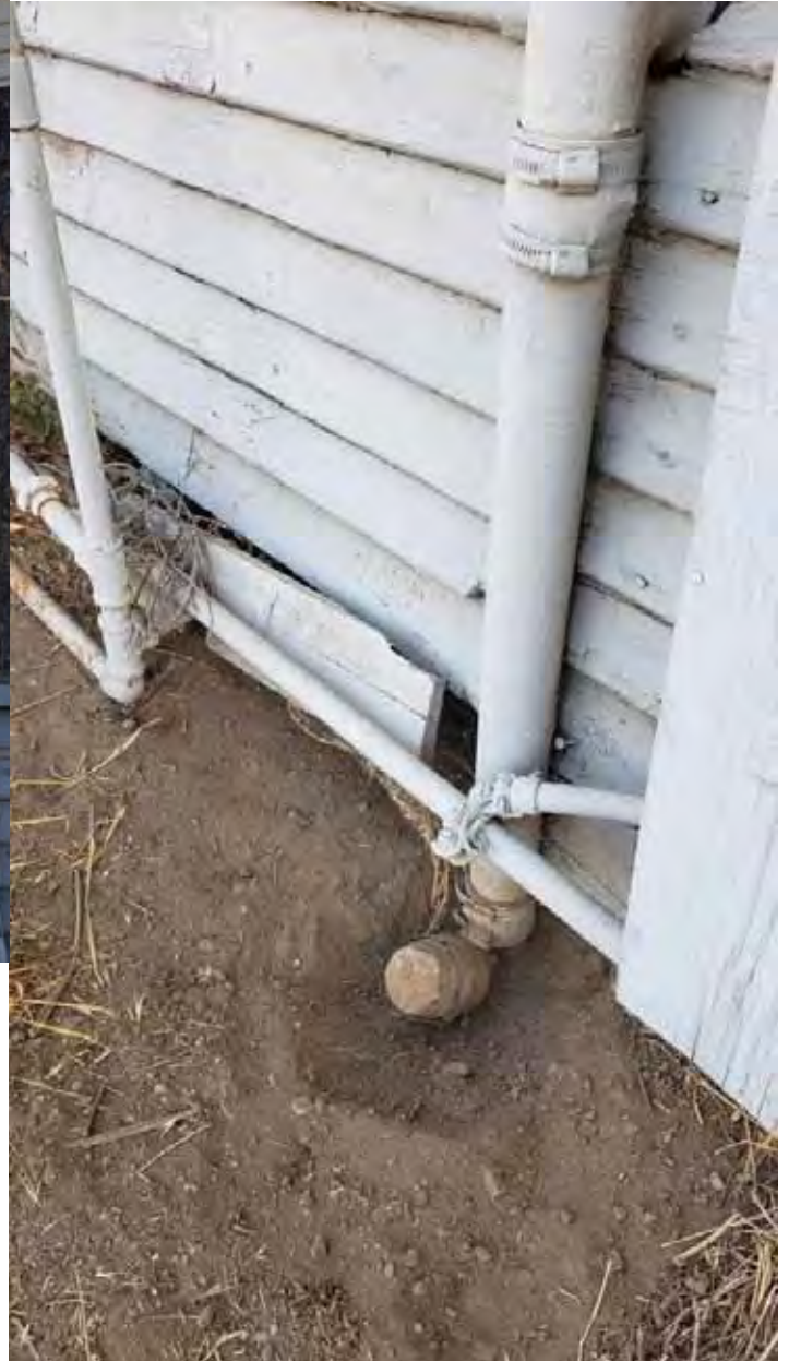
Photo 16: Base of vent line with apparent fill pipe to heating oil tank.
