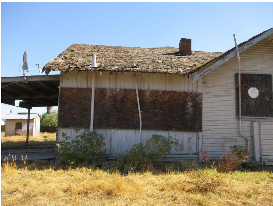
Figure 4. West elevation, showing the hipped gable form clad in vertical wood boards, facing east.
