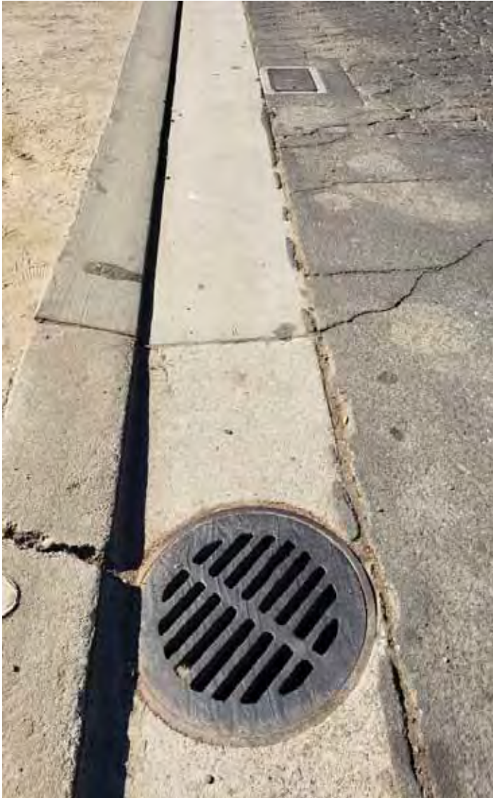
Photo 31: Storm water catch basin along Irwin Avenue, near northwest corner of property.
