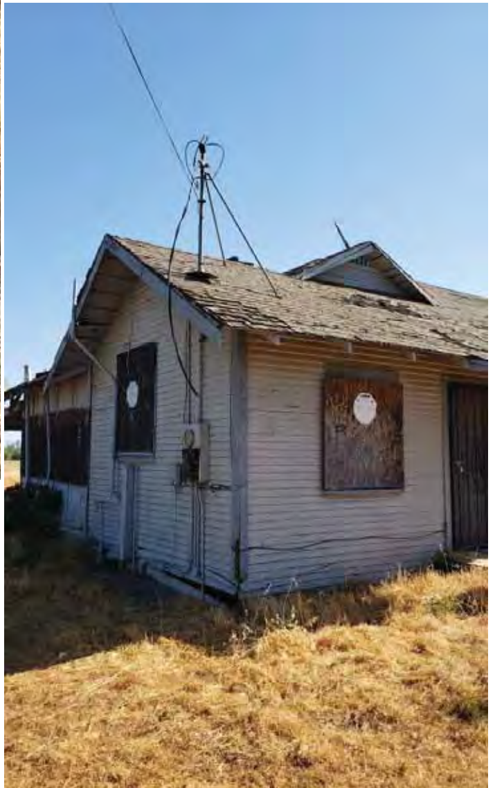
Photo 12: Southwest corner of boarded up residence on APN 225-070-320. Note vent lines on west side of building.
