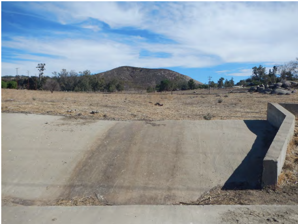
Photograph 4 – View of the concrete apron associated with the unnamed jurisdictional drainage that is offset a minimum of 200 feet from (north of) the Major Use Permit (MUP) area, facing east.
