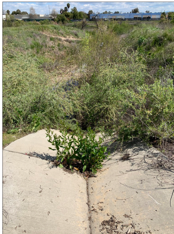
Photograph 8: Photograph of Drainage E located in the central portion of the study area, facing northeast.
