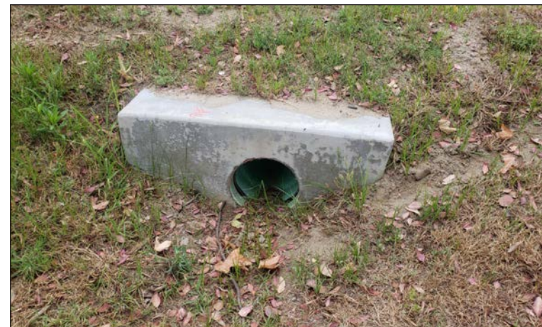
Photograph 4: View of an open culvert in the center of the project, facing west.
