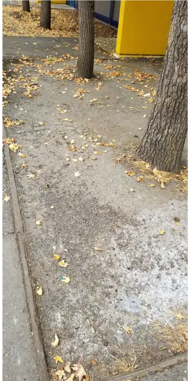
Figure 6: Compacted soils around liquidambar trees.
