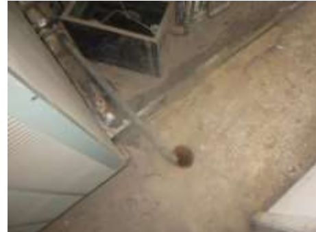
FLOOR DRAIN/SUMP IN BASEMENT MECHANICAL ROOM
