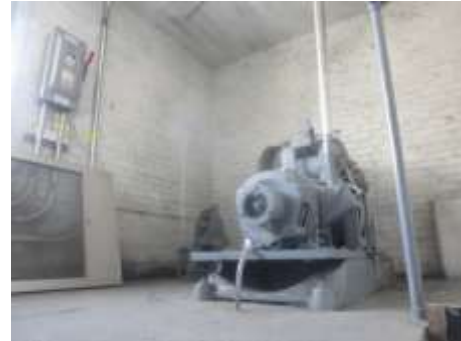
ROOFTOP PENTHOUSE ELEVATOR MECHANICAL ROOM
