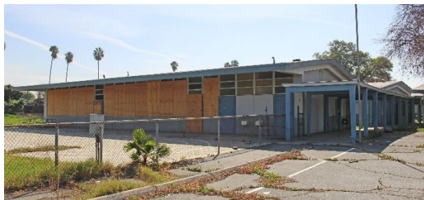
Figure 13: Building G. South elevation above and north and west elevation below. 2020. Source: GPA.
