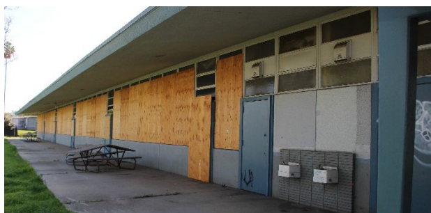
Figure 11: Building E. South and east elevation above and north elevation below. 2020. Source: GPA.
