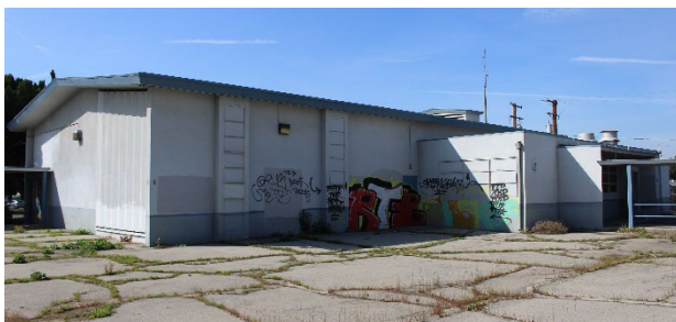
Figure 8: Building B. South and west elevation above and north and east elevation below. 2020. Source: GPA.
