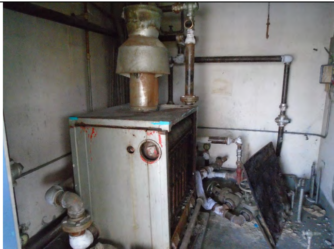
Mechanical room interior
