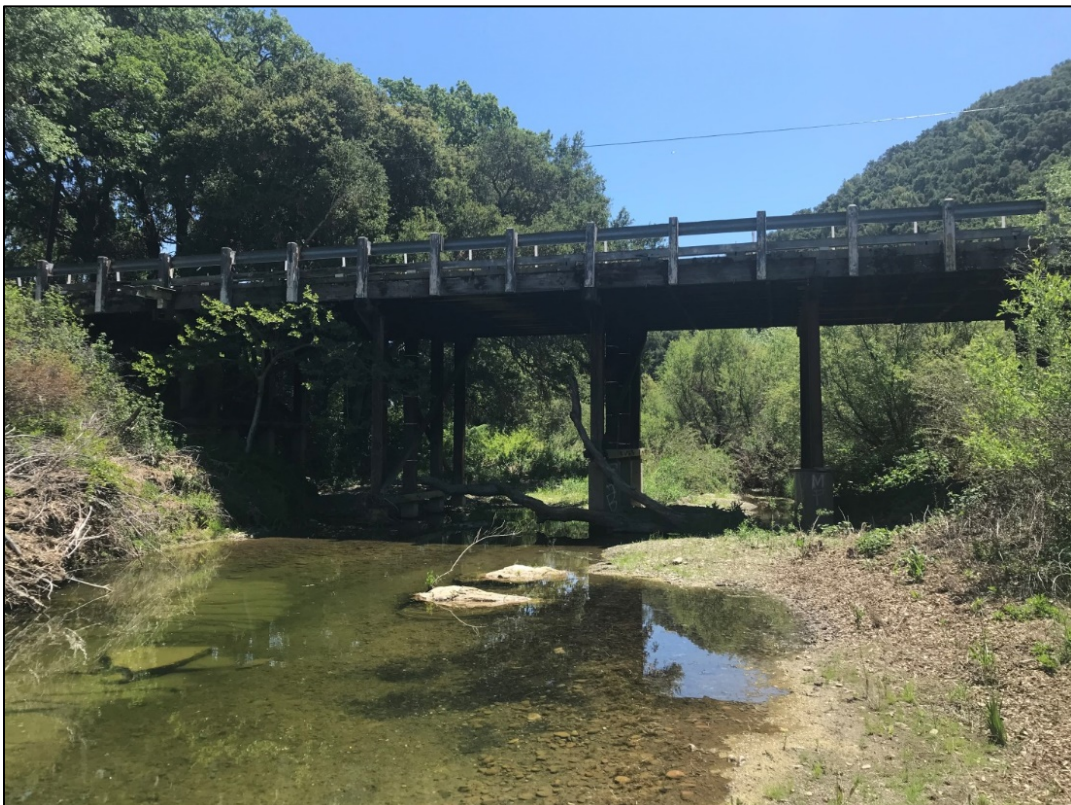
Photo 4. Jack Creek Road Bridge over Paso Robles Creek, facing east. Conditions are expected to be much drier than this during construction. Photo taken May 4, 2021.
