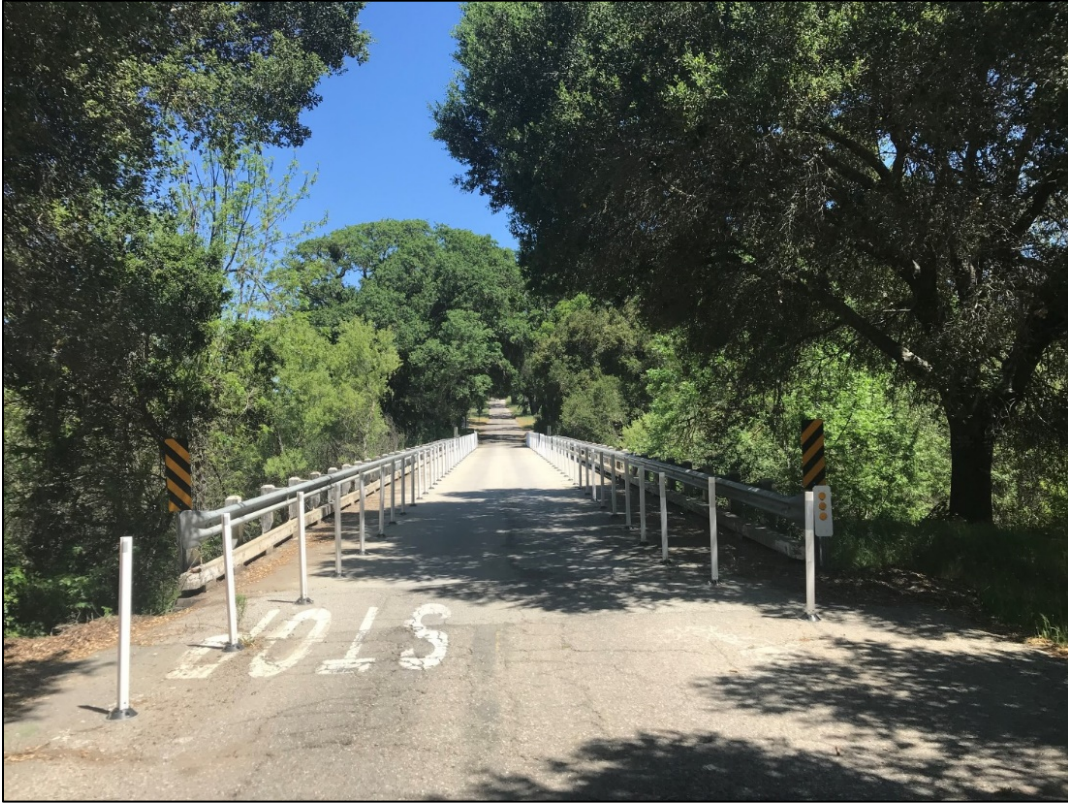
Photo 1. Jack Creek Road Bridge over Paso Robles Creek, facing northeast. Photo taken May 4, 2021.
