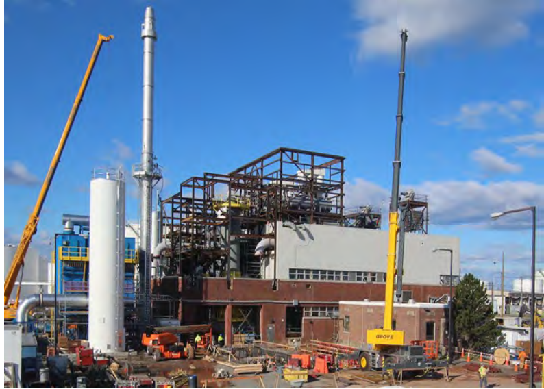
Photograph 2-3 Biosolids Fluidized Bed Gasification Facility in Linden New Jersey
