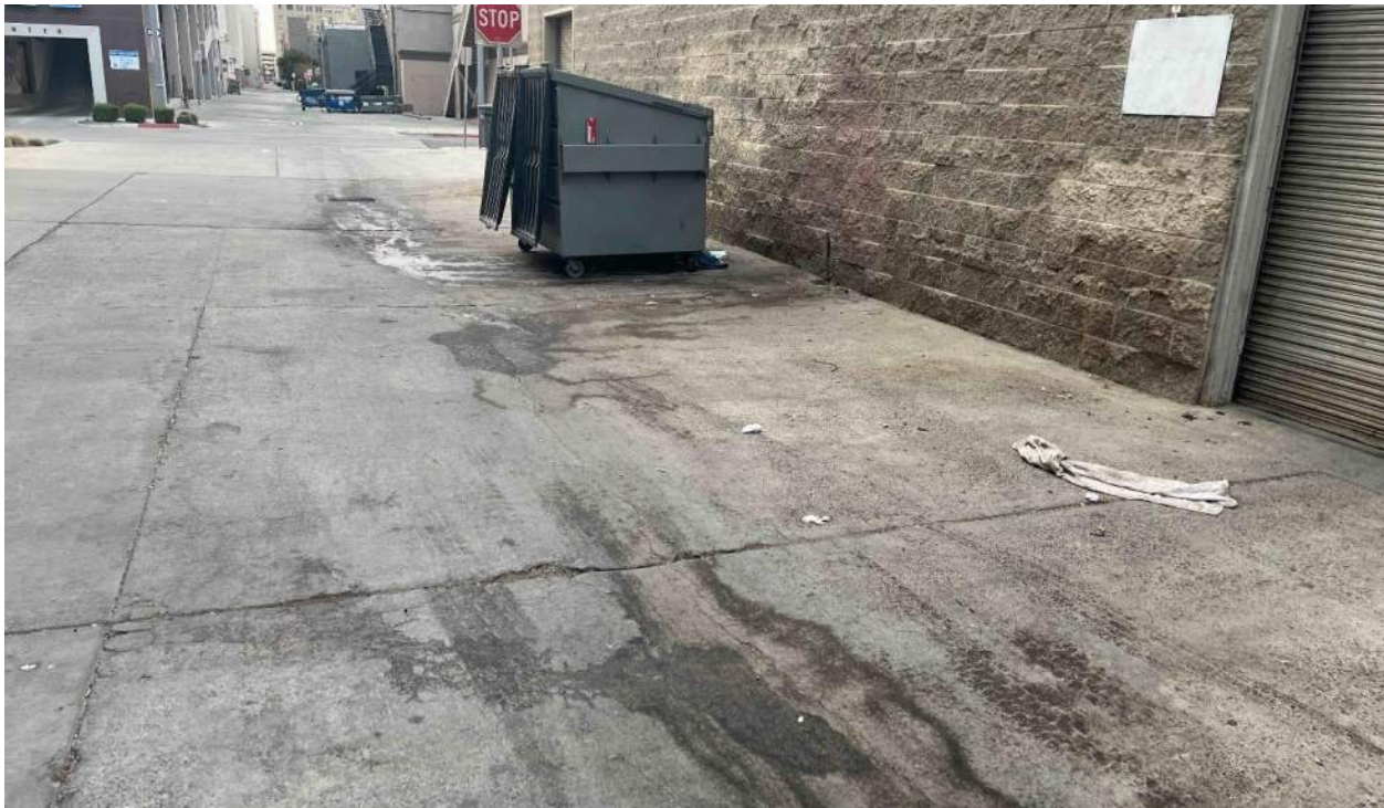
Figure 10 Pavement Staining within Alleyway South of Merced Street, Facing Southeast
