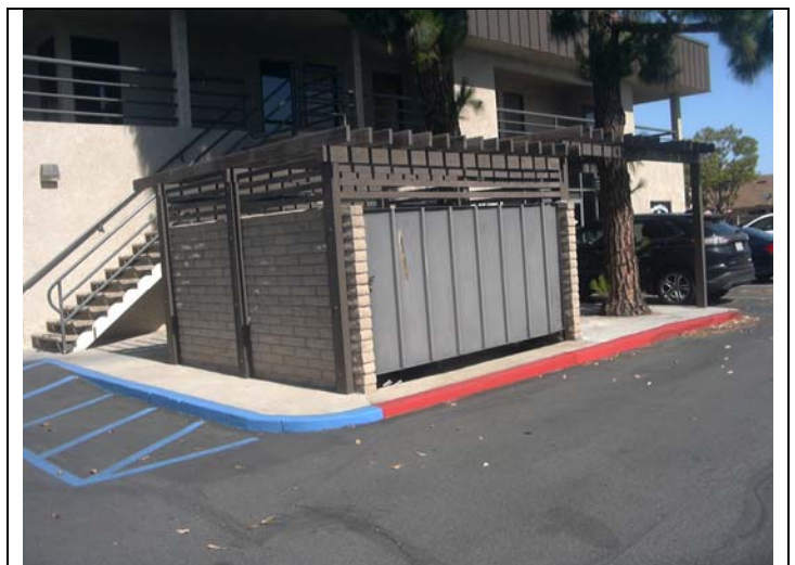
6. View of high-voltage transformer enclosure.
