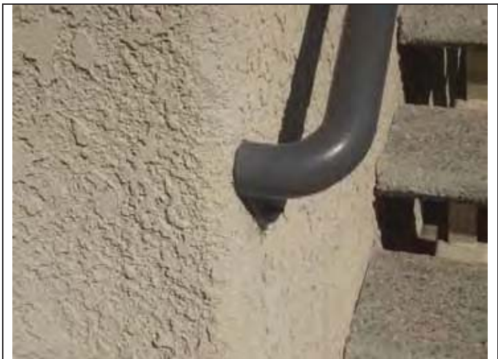
70. Handrail does not extend 12 inches horizontally beyond stairs.
