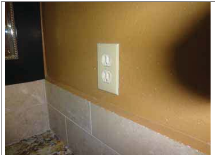
72. A non GFCI electrical outlet located adjacent to one of the common restroom lavatories.
