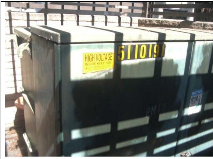
7. View of the high-voltage transformer at the subject property.
