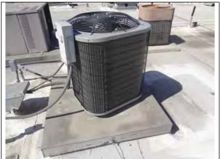
46. Typical condenser component of a split system HVAC unit.
