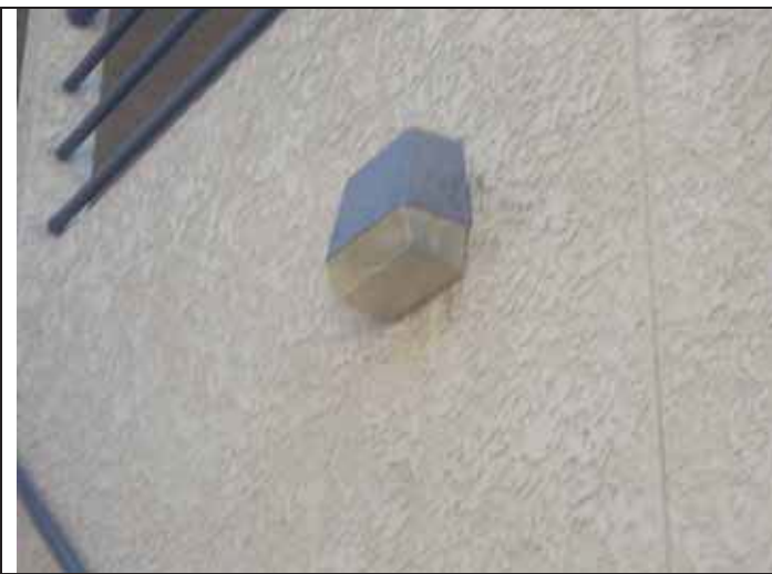
21. Typical façade-mounted exterior lighting fixture.
