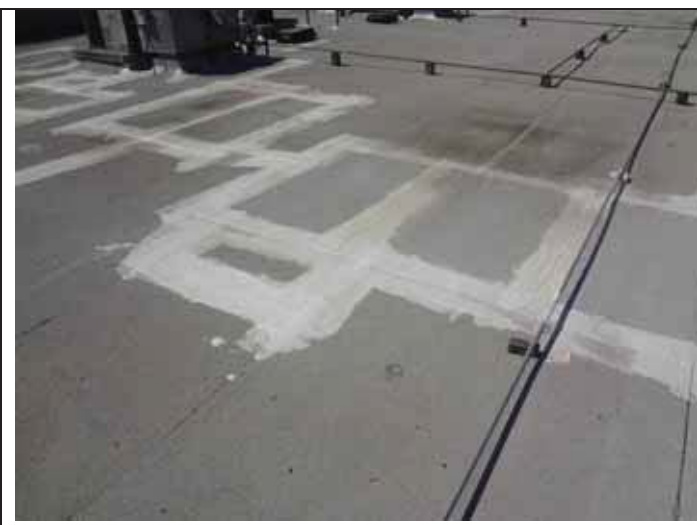
35. Example of past roof repairs on the 10221 Building.
