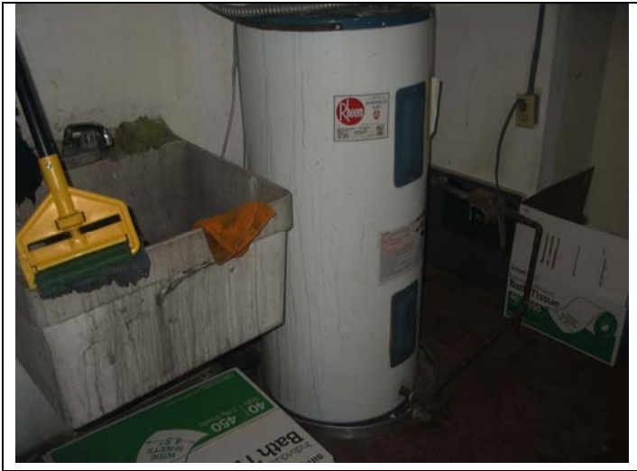
19. View of an electrical water heater at the subject property.
