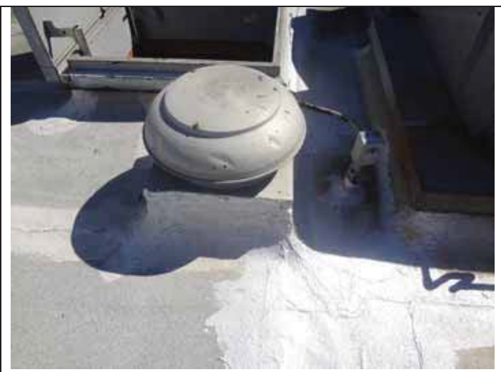
47. Typical common restroom powered exhaust fan.
