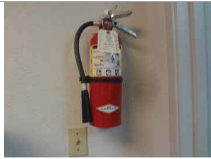
53. Typical portable fire extinguisher within a tenant space.
