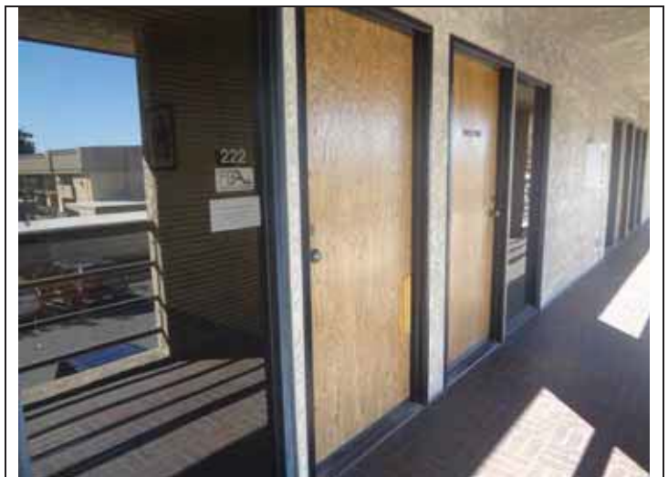
40. Typical storefront and wood entrance doors to the second floor tenant spaces.
