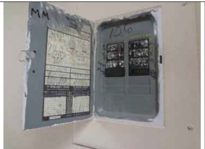
52. Typical electrical sub-panel within a tenant space.
