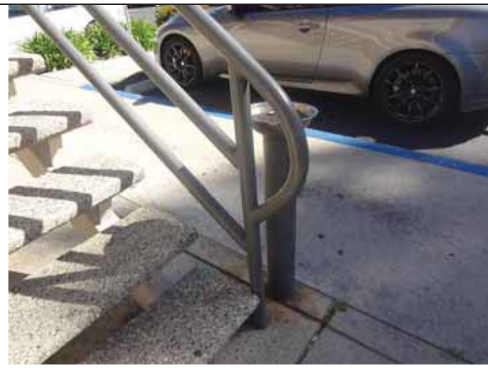
69. Handrail does not extend 12 inches horizontally beyond stairs.
