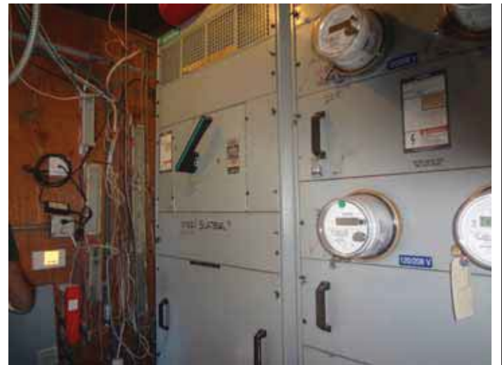
50. One of the main electrical switchgear, meters and distribution panels.
