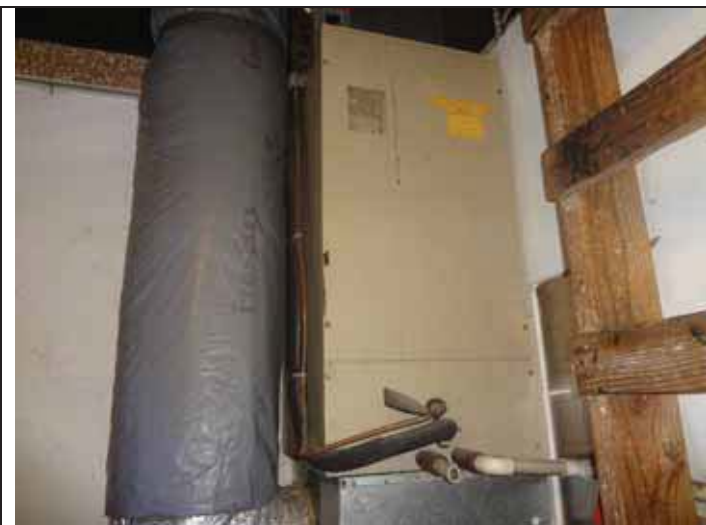
45. Typical interior fan coil of a split system HVAC unit.
