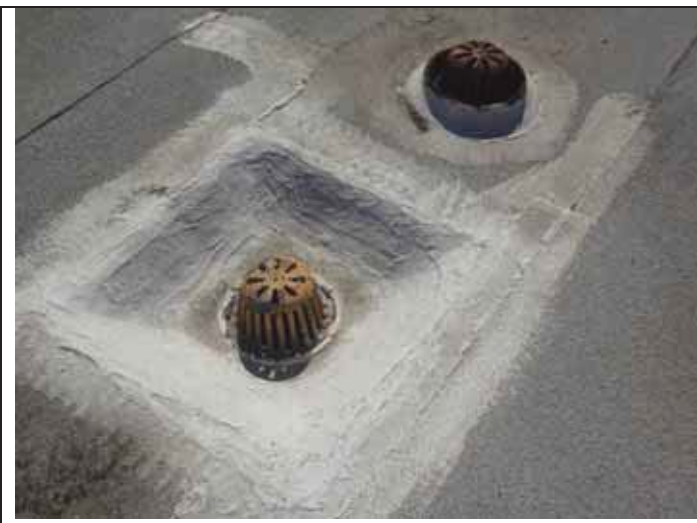
33. Typical primary and overflow roof drains.
