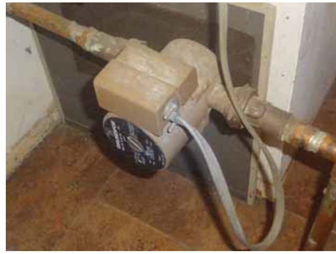
49. Electric domestic water circulation pump.
