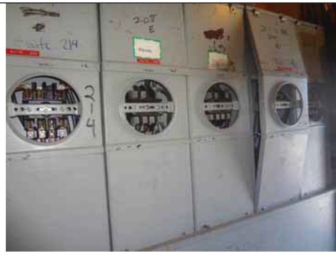
71. Electrical meter openings that are not blanked off.
