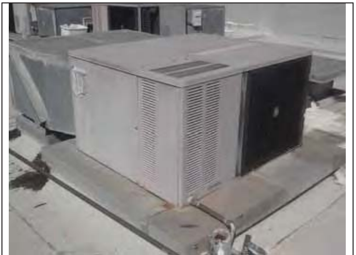
44. Typical roof mounted HVAC heat pump.
