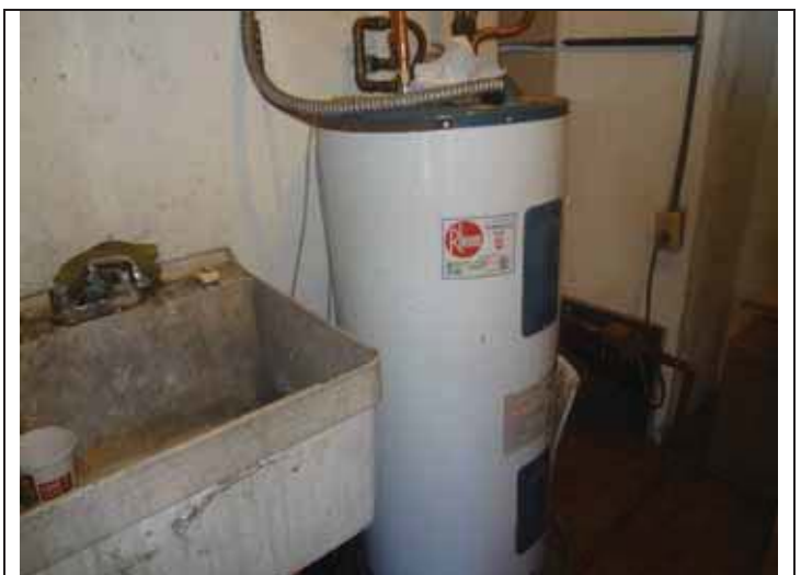
48. One of two domestic water heaters.
