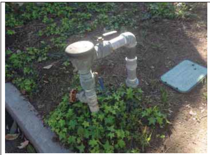
27. Domestic water service and backflow preventer.
