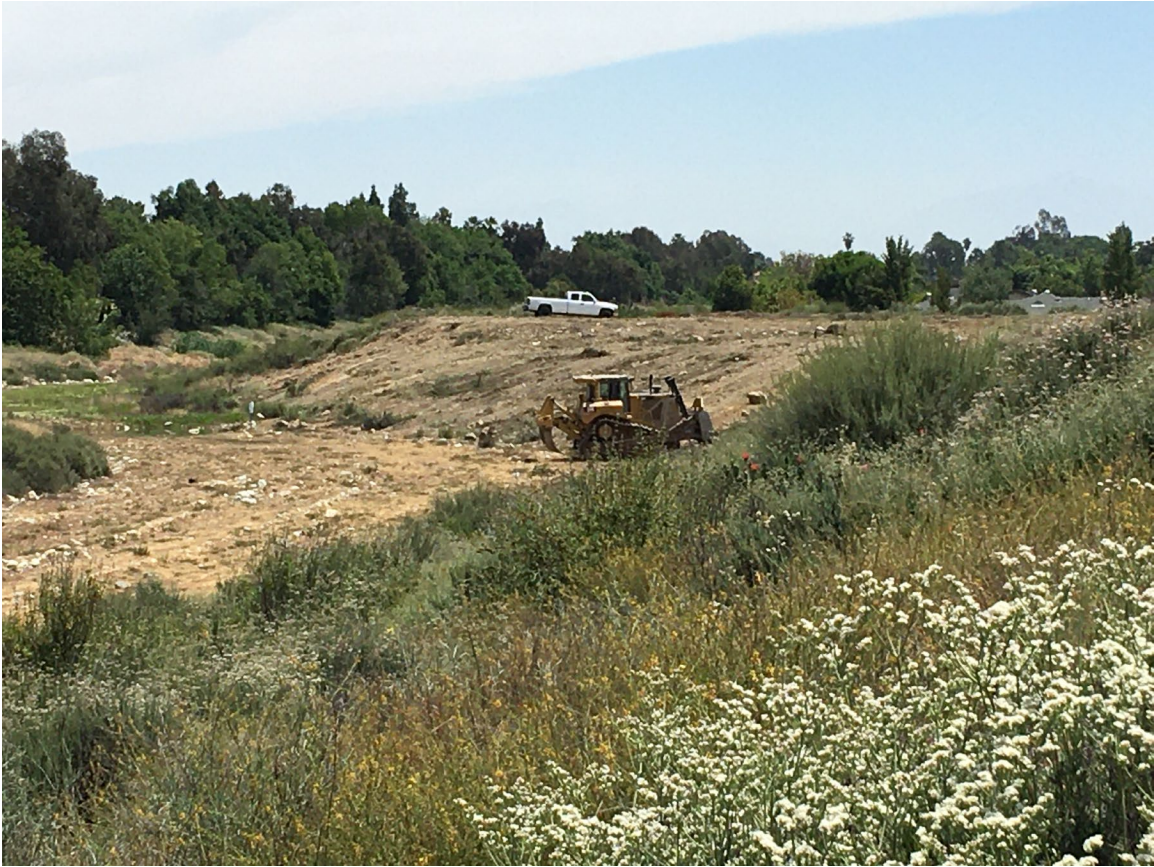
West side of basin looking north east. South slope of basin pictured during bulldozing. Photo taken May 14, 2020.
