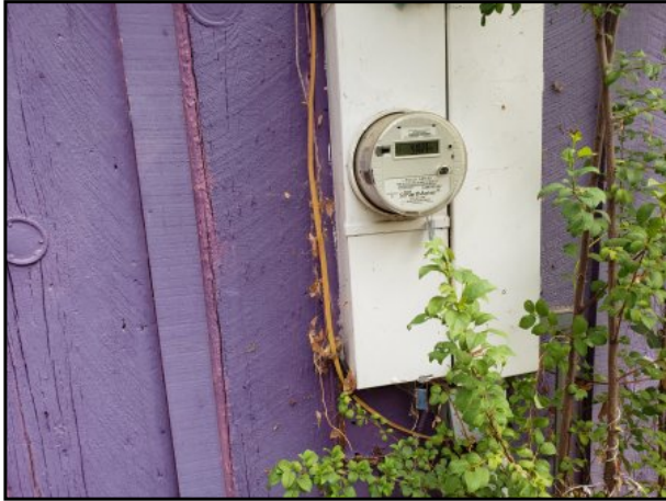
5 : Photograph of PG&E electric meter located on south side of residential dwelling.
