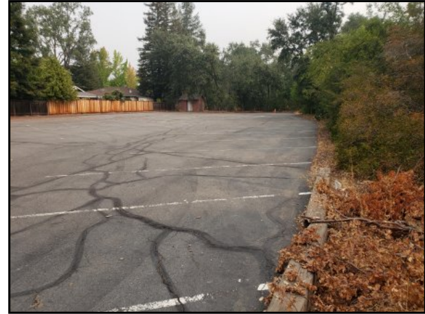
2 : Photograph of Calistoga Seventh Day Adventist Church parking lot area located west of subject property.
