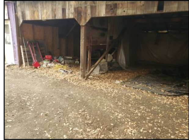
6 : Photograph of wood garage attached to the north side of residential dwelling.
