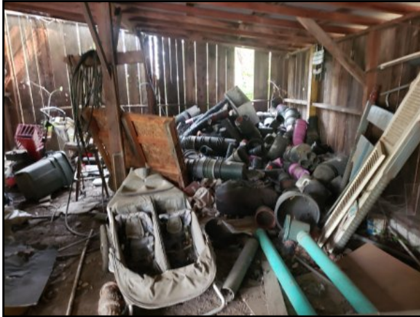
9 : Photograph of general trash and debris stockpiled in the wood shed structure.
