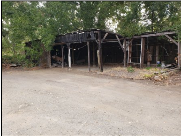
7 : Photograph of fire-damaged wood shed structure located in southwest section of subject property.
