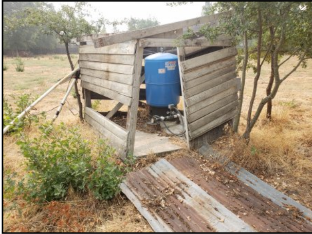
13 : Photograph of abandoned water well area located in central section of subject property.
