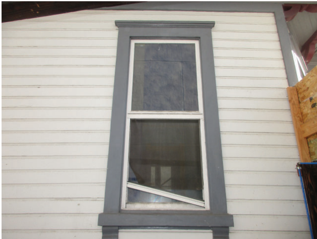
Figure 3-15: Detail photo showing a typical replacement clad wood window with dual glazing and vinyl window screens.
