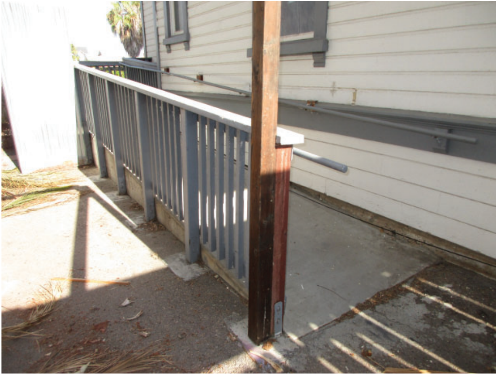
Figure 3-13: Looking northwest at the accessibility ramp located at the south facade. The ramp is a combination of cast-in-place concrete and OSB wood boards.
