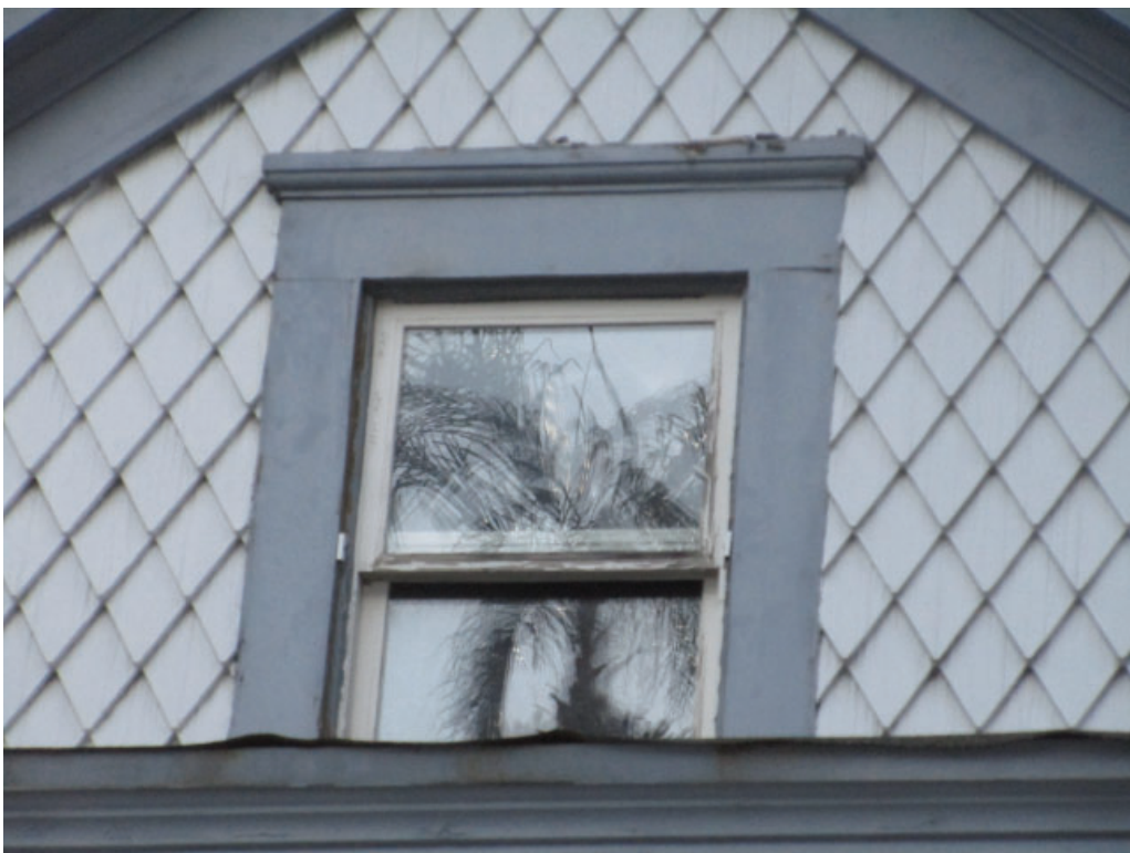
Figure 3-6: Looking west at the gable end of the east facade showing the diamond shaped wood shingles and replacement double hung window.
