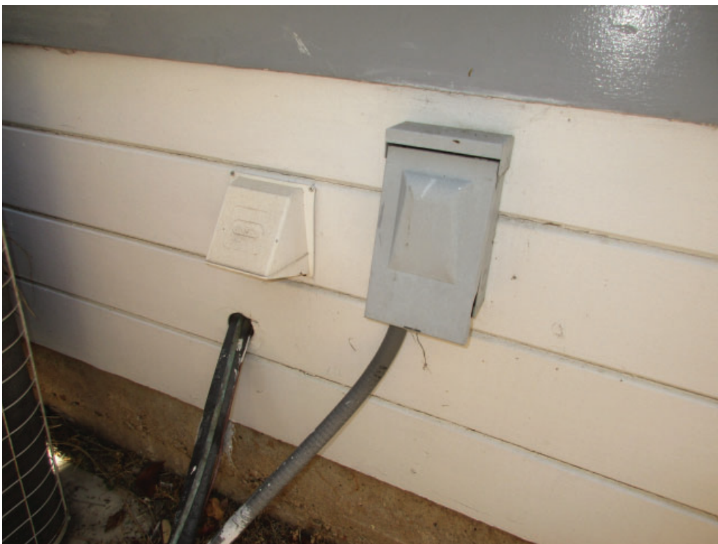
Figure 3-18: Detail photo showing some of the utility equipment installed at the base of the north facade.
