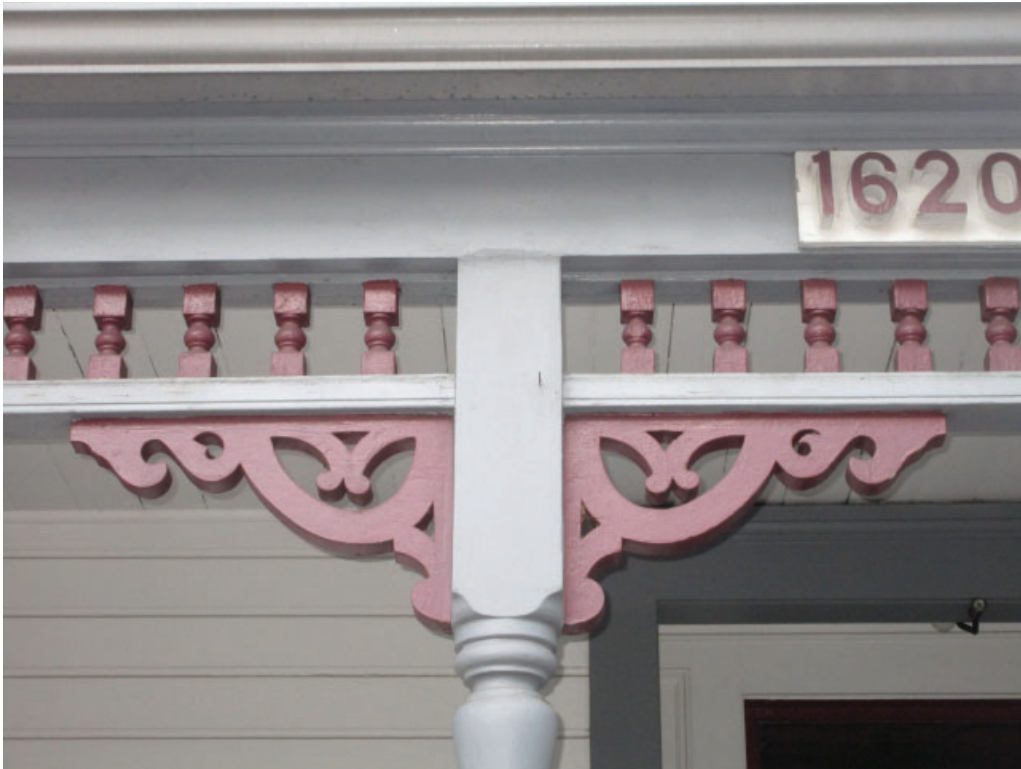
Figure 3-7: Detail photo showing the decorative wood spindlework and decorative column brackets at the front porch.
