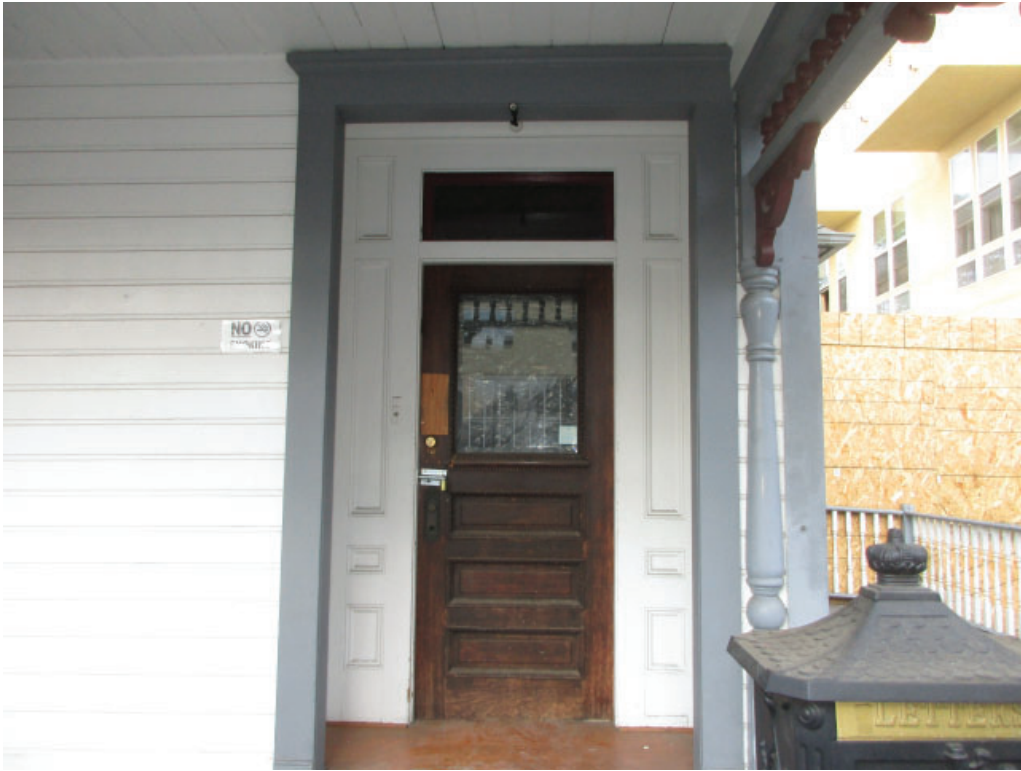
Figure 3-9: Detail view showing the original three panel entry door with glazed lite and fixed wood transom window above. The original door hardware is missing.
