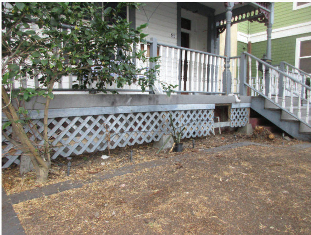
Figure 3-10: Looking northwest at the front porch, front porch stairs and railing. The front porch is non-historic and has been replaced with OSB boards.
