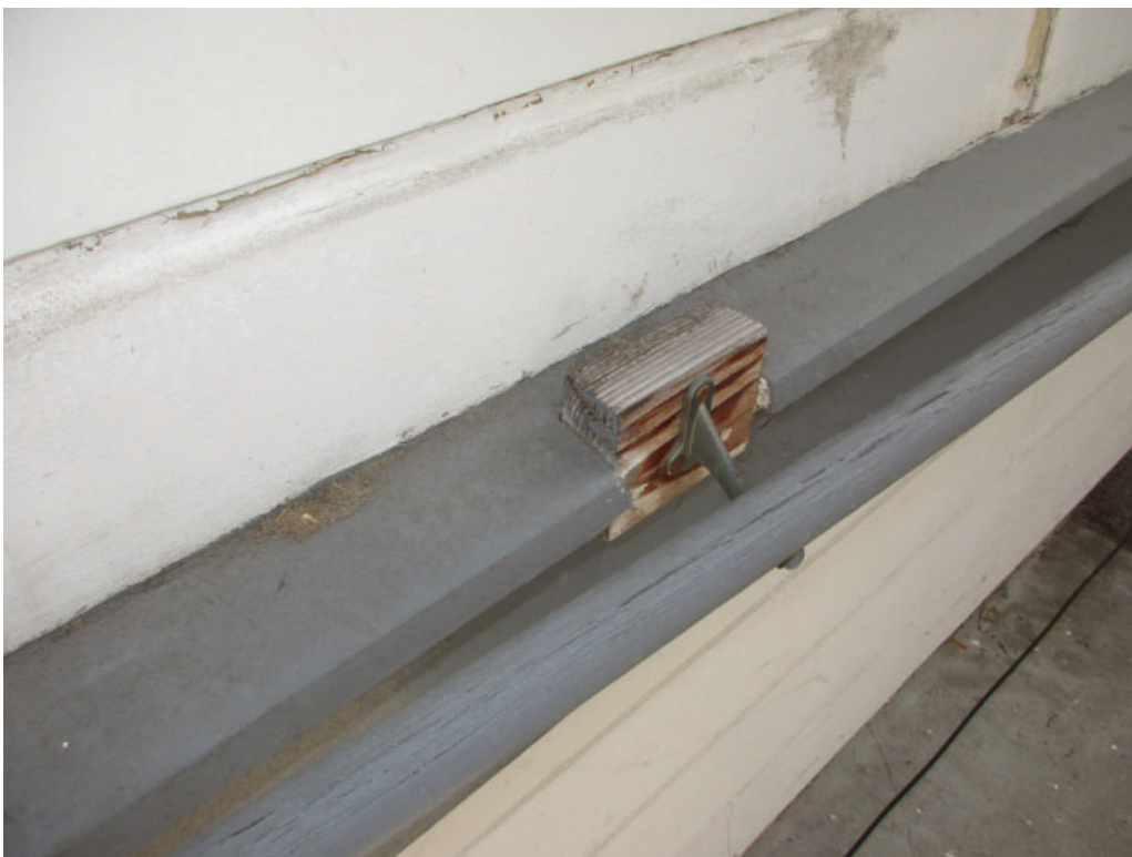
Figure 3-14: Detail photo showing the impact to the base trim boards from the accessibility ramp handrail attachments.
