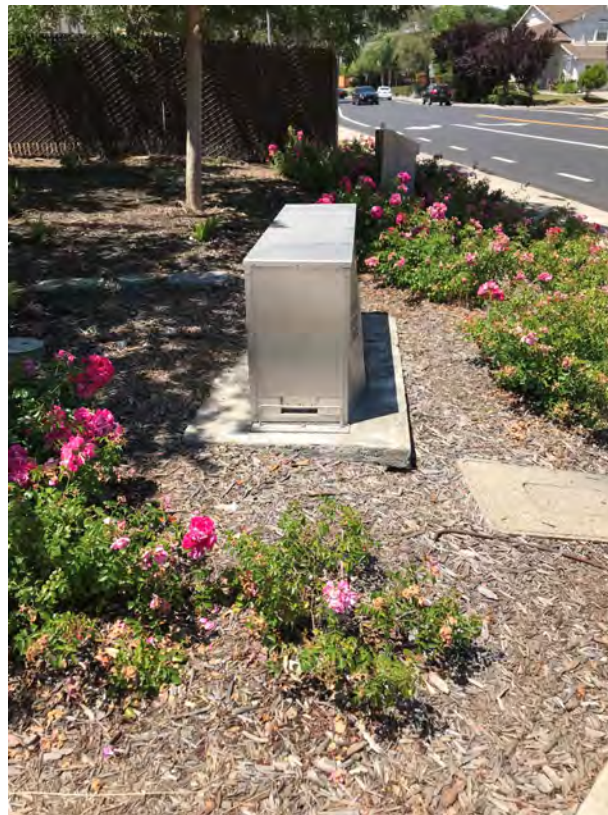
Photo 24 – Utility vaults corner of West Side Drive and San Ramon Valley Blvd.
