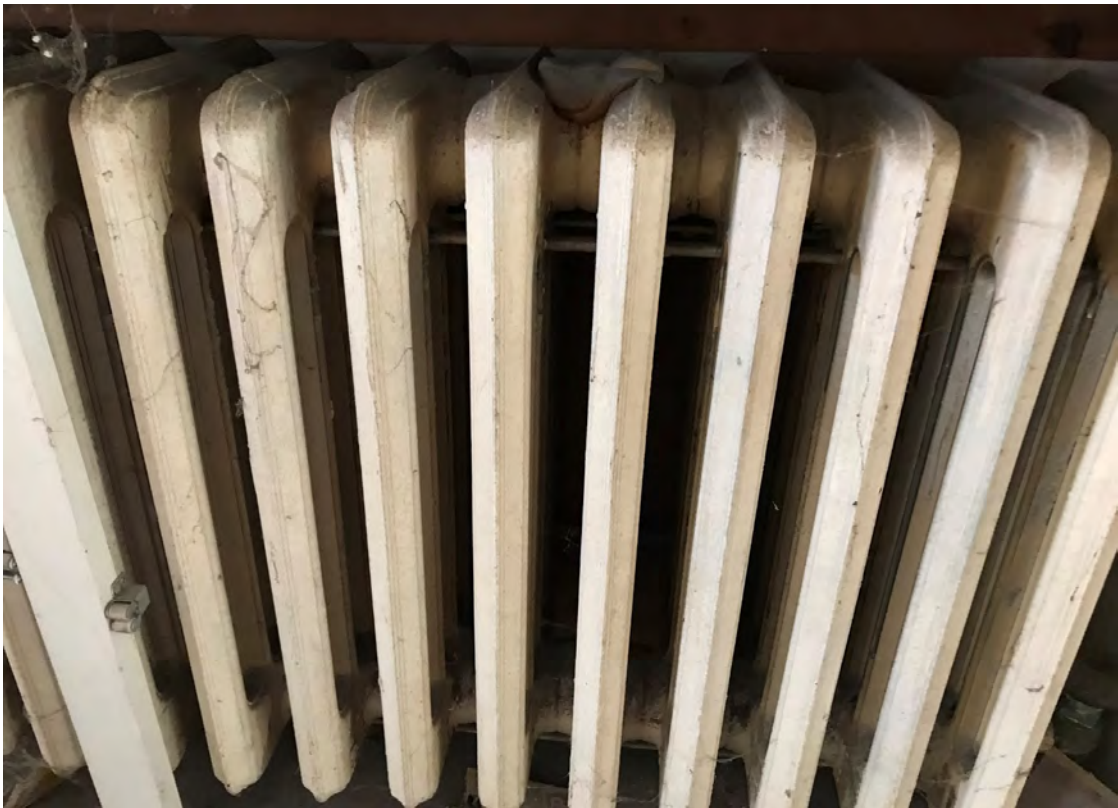
Photo 2 – House, radiant heater, east wall 1st floor
