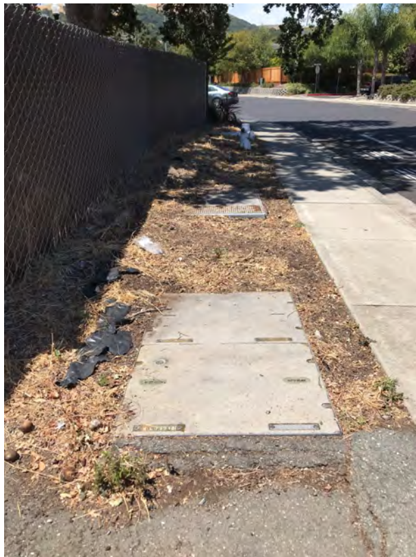
Photo 22 – Utility vaults (1), adjacent to east fence, West Side Drive
