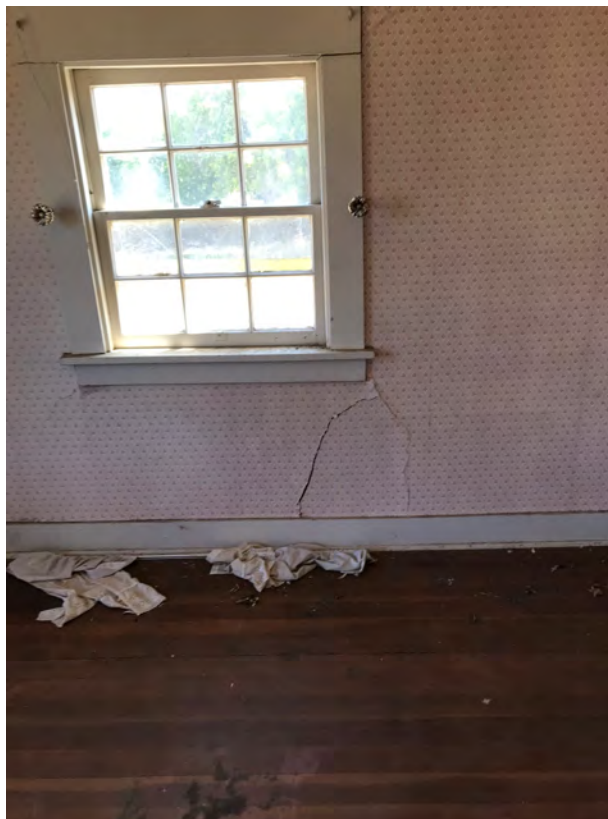
Photo 6 – House, East wall, 2nd floor, broken drywall
