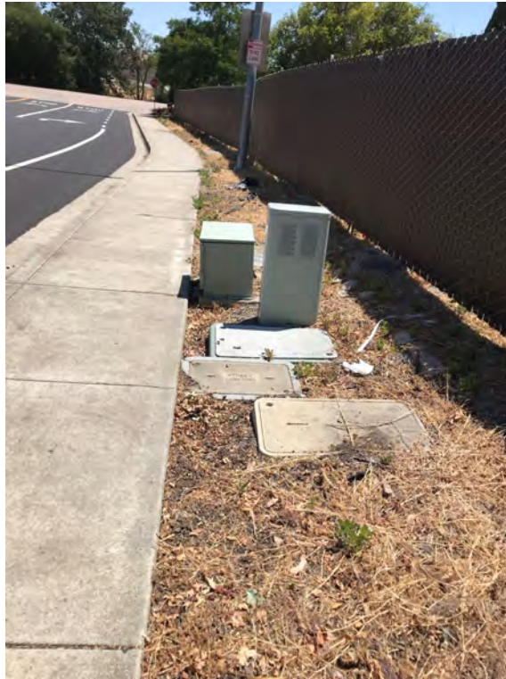
Photo 23 – Utility vaults (2) adjacent to east fence, West Side Drive
