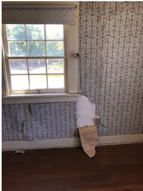
Photo 8 – House, east wall, 2nd floor, peeling wall paper
