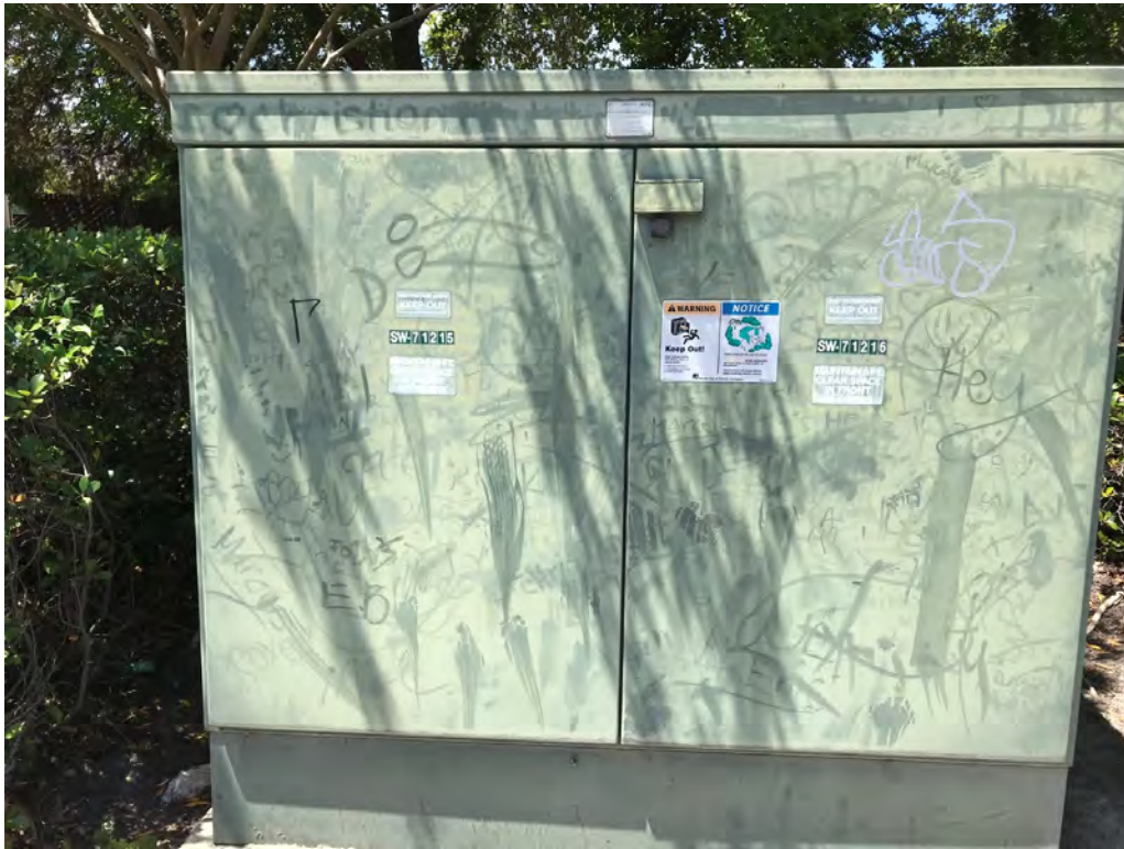
Photo 25 – San Ramon Valley Blvd, high voltage vault adjacent to east fence
