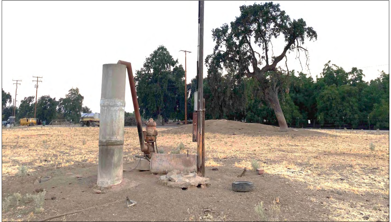
Figure 7. Photograph of the western border of the well installation site, looking northwest, showing the previous well, pump, and electrical pole, and the valley oak and another earthen mound at the northwest corner of the well installation site.
