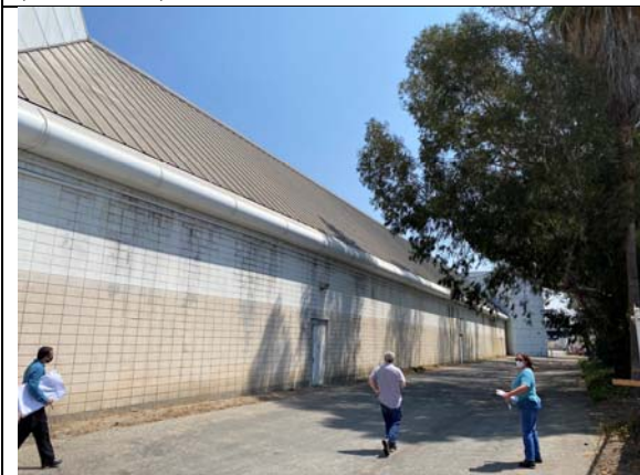
West portion of side (south) façade with stair volume in background, view east (Bastien, 2020)
