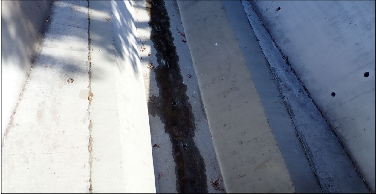
Photograph 2. View of the extent of water flow and water staining in the creek channel during the site visit. Photograph taken on June 1, 2021.
