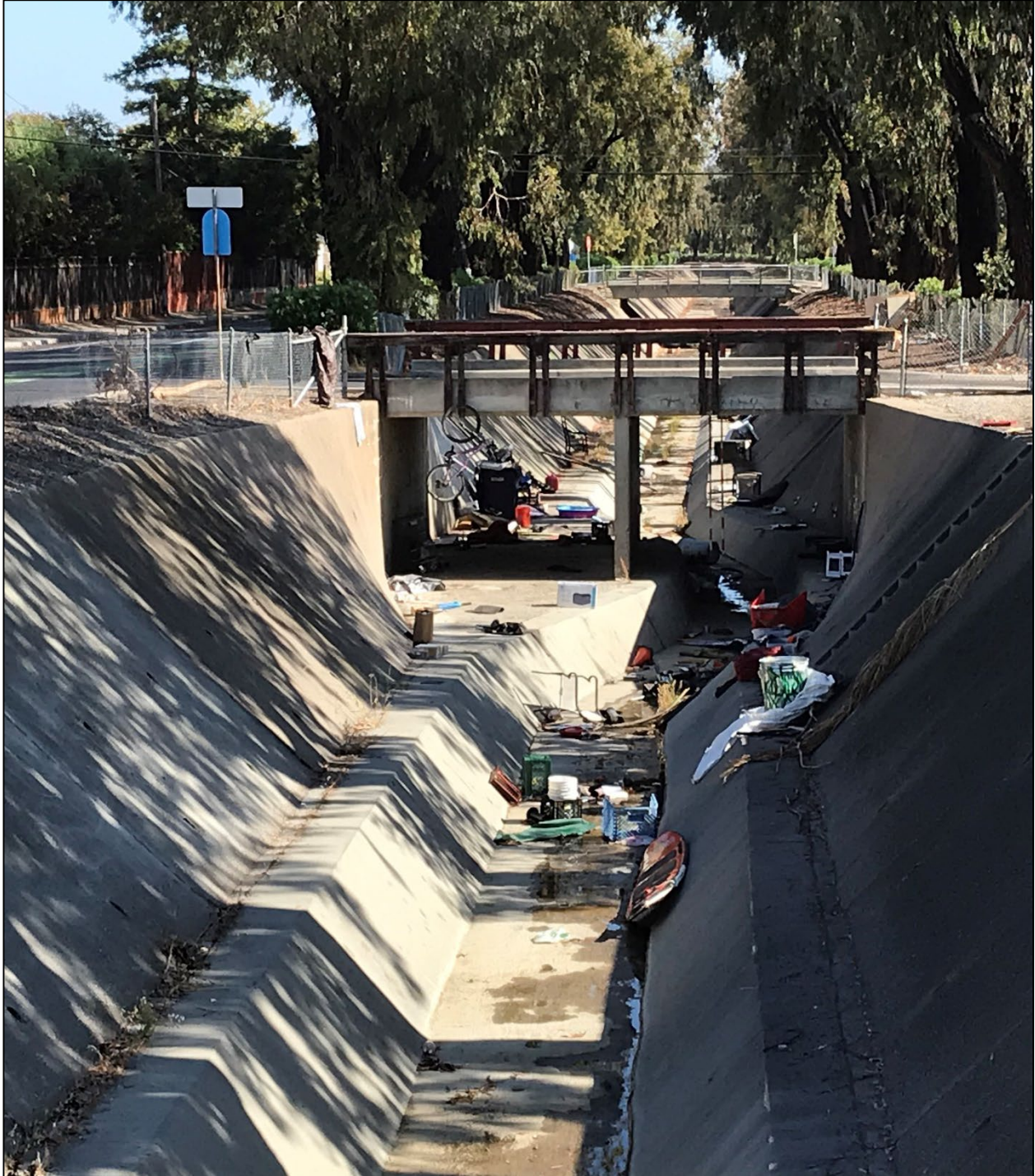
Photograph 1: View of the bridge proposed for removal over Calabazas Creek taken looking north from the intersection of El Camino Real and Calabazas Boulevard. Photograph taken on June 2, 2021.
