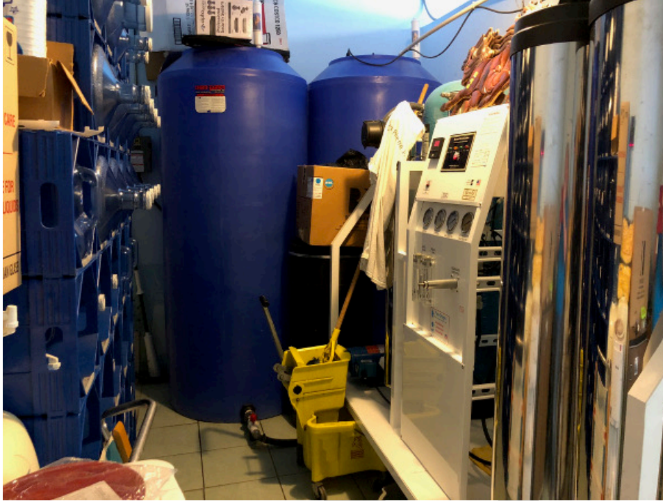
Photograph 11. Water purification system within tenant unit.
