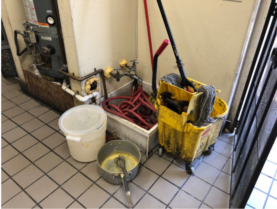
Photograph 37. Closer view of cleaning supplies and drain on north side of structure.
