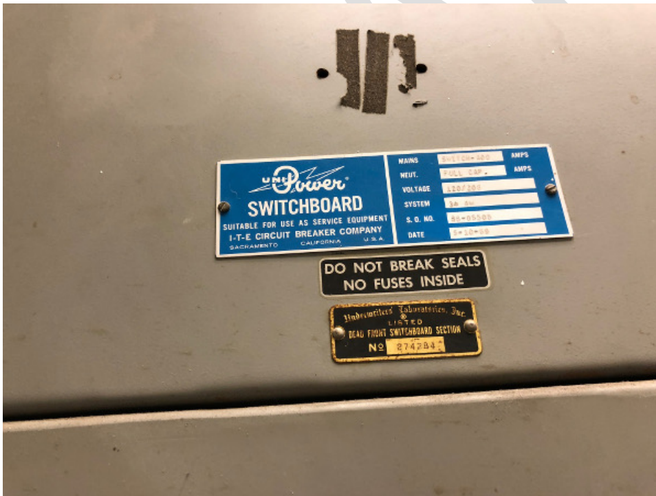
Photograph 6. Electrical switchboard, dated 1969.
