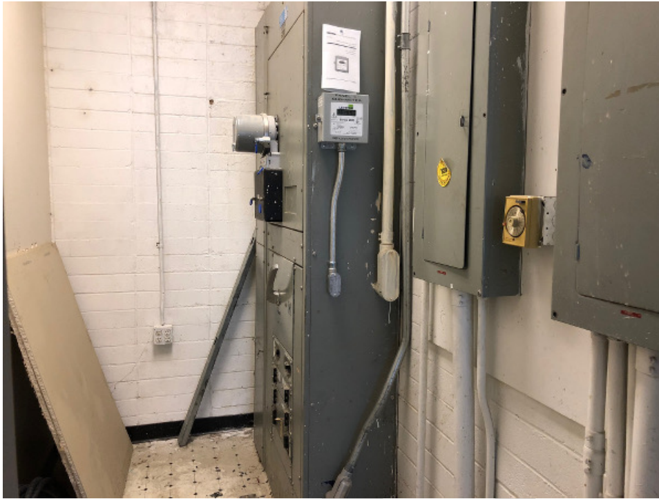
Photograph 5. Electrical room in northwest corner of shopping center structure.
