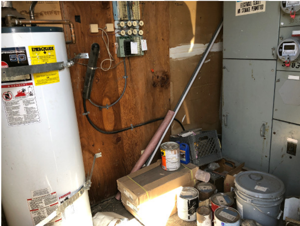
Photograph 51. Electrical and water heater property management space, also storage location of paints and maintenance supplies, located along eastern side of shopping center structure.
