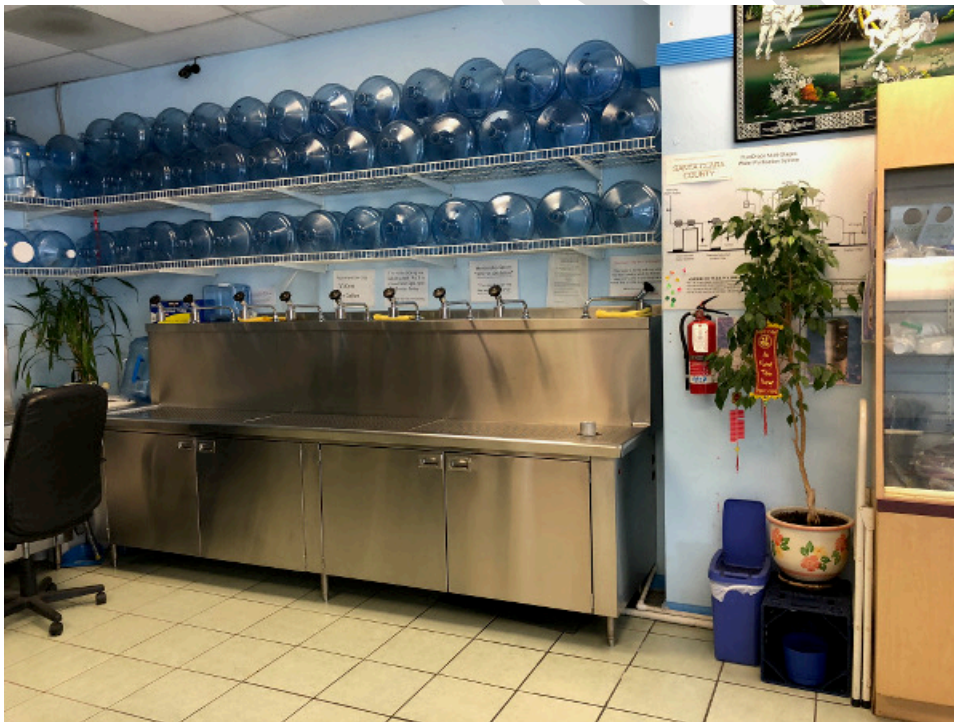
Photograph 10. Purified water dispensing equipment within tenant unit.
