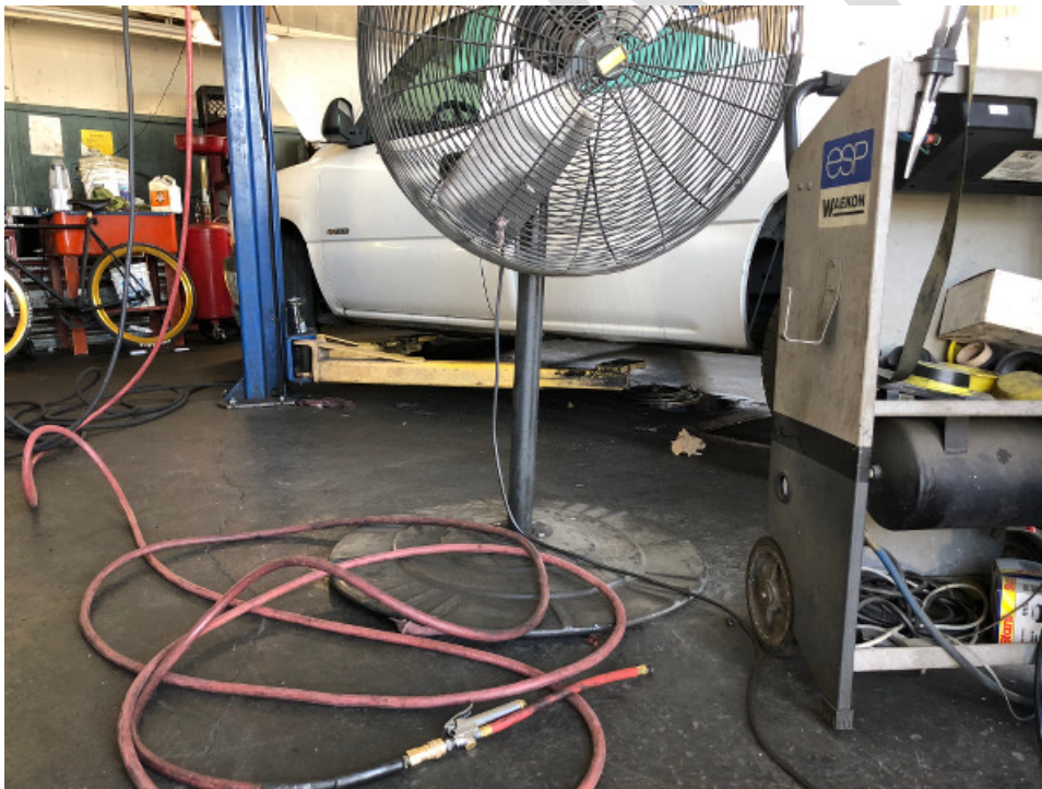
Photograph 71. Vehicle lift system, apparent hydraulic lift.
