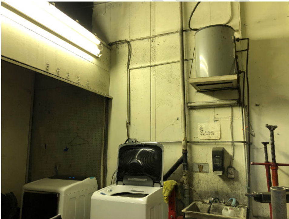
Photograph 69. Additional view of washer, dryer, and water heater equipment in northwest corner of automobile service structure.
