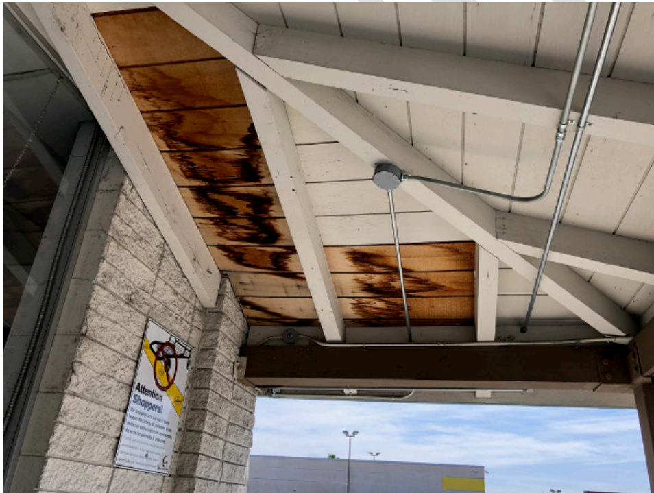
Photograph 49. Apparent damage to roof at southeast corner of shopping center structure.
