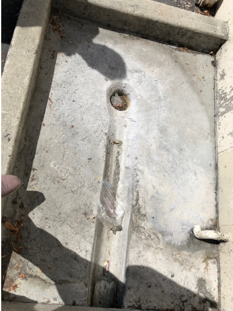
Photograph 43. Exterior containment and drain, reportedly serving the washer and dryer shown in photo 41.
