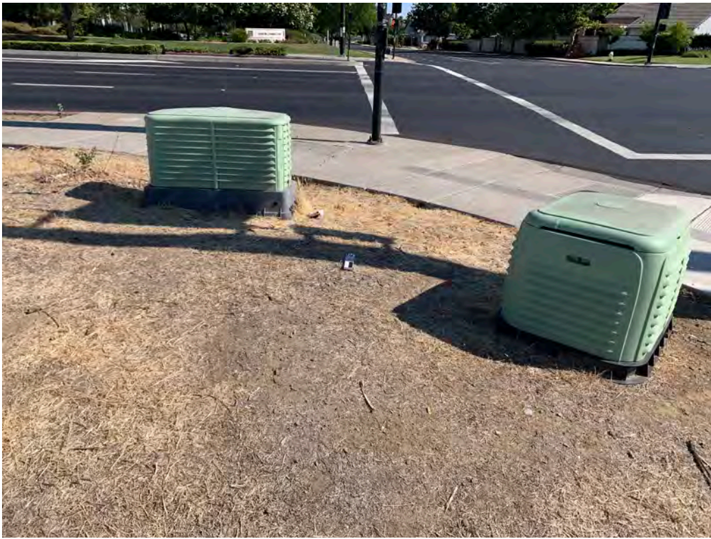
Photo 7: Overview of telecommunications boxes (disturbance), facing north
