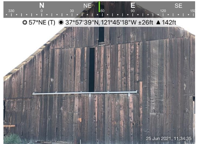
Photo 6. Missing boards on the west side of the old barn.
