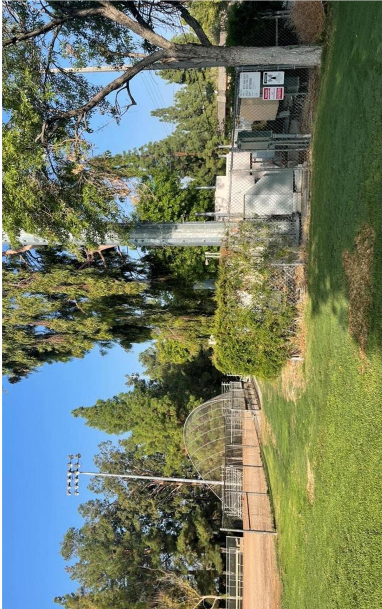
Figure 8 Photo 4 View of Existing Cell Tower at Project Site, View to the West
